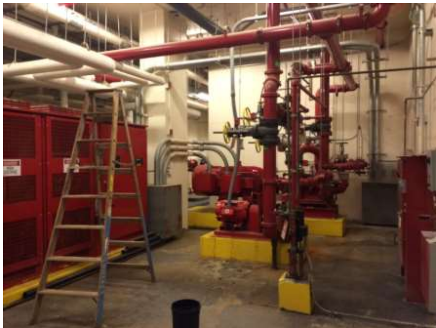
Photo 12: Surface cover in Site fire pump room.
