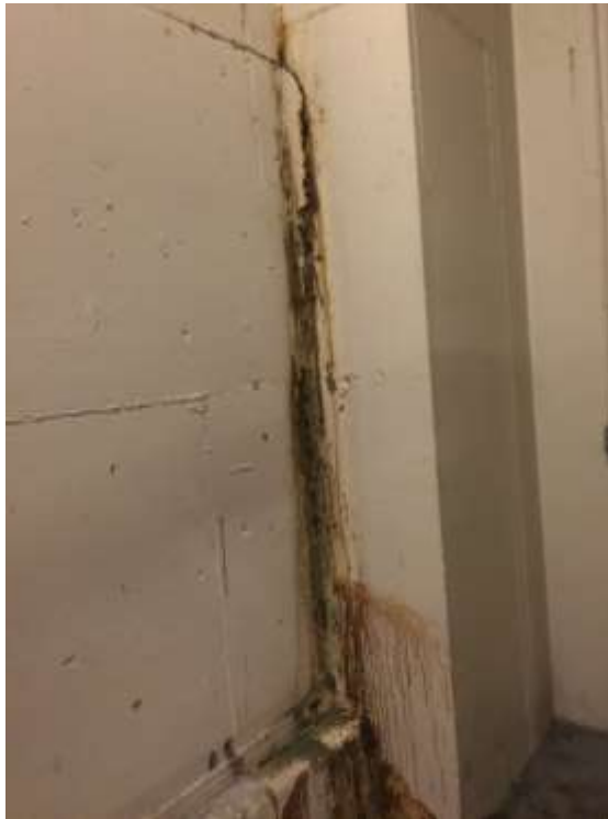
Photo 3: Seepage on the wall of the sub-cellar level on August 23, 2016.
