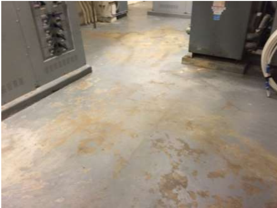
Photo 5: Surface cover in Site compactor room.
