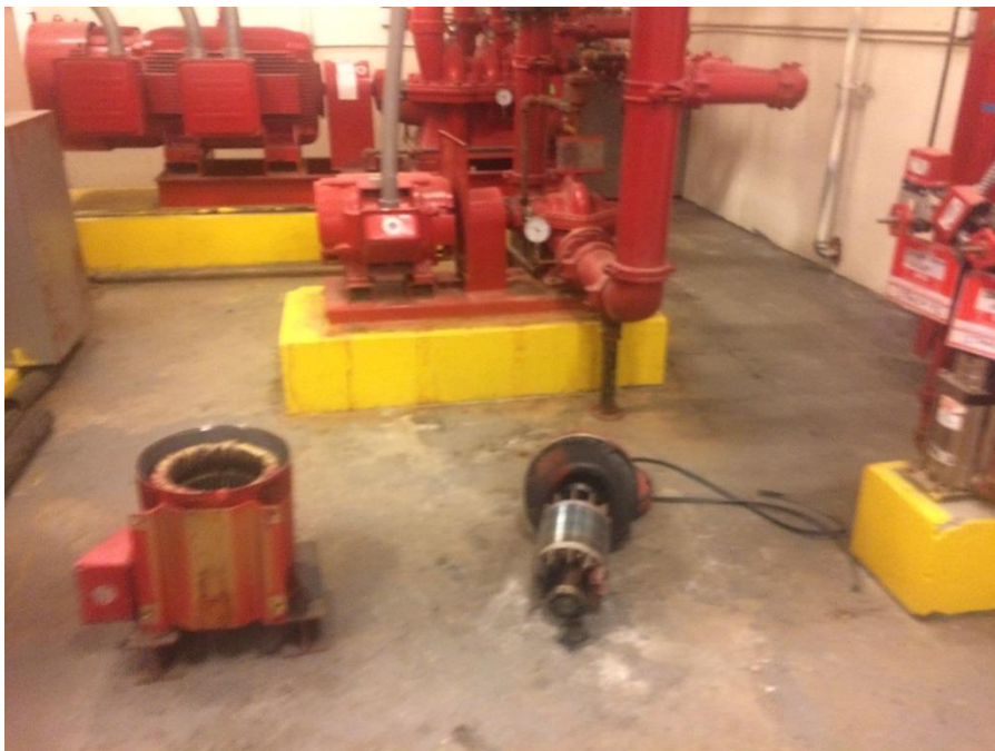
Photo 12: Surface cover in Site fire pump room.
