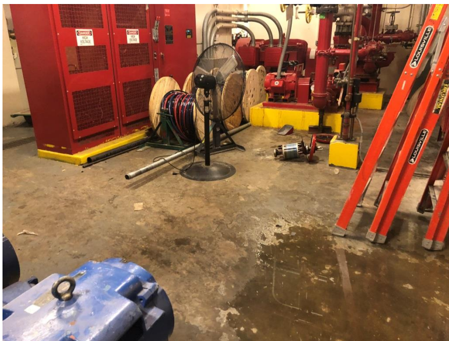
Photo 14: Surface cover in Site fire pump room.
