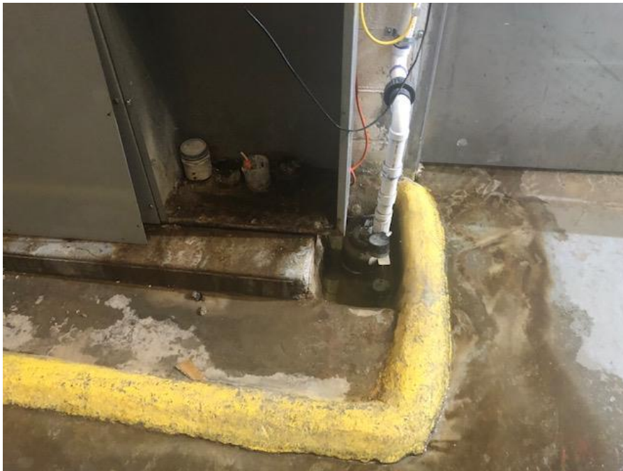
Photo 2: Water intrusion and sump pump in the Site electrical services room
