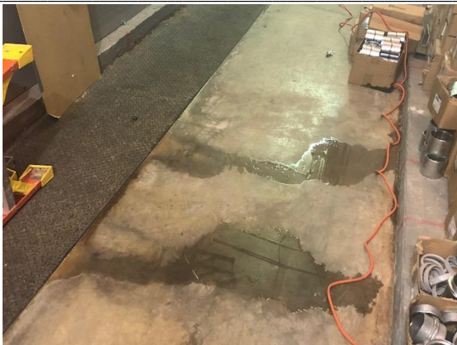
Photo 3: Water intrusion in the Site electrical services room.
