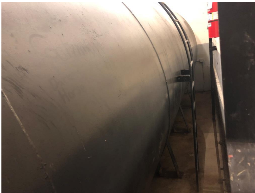
Photo 10: Water intrusion through the surface cover of the Site AST room.
