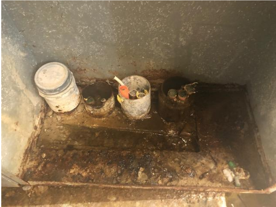
Photo 1: Water intrusion through conduit in the Site electrical services room.
