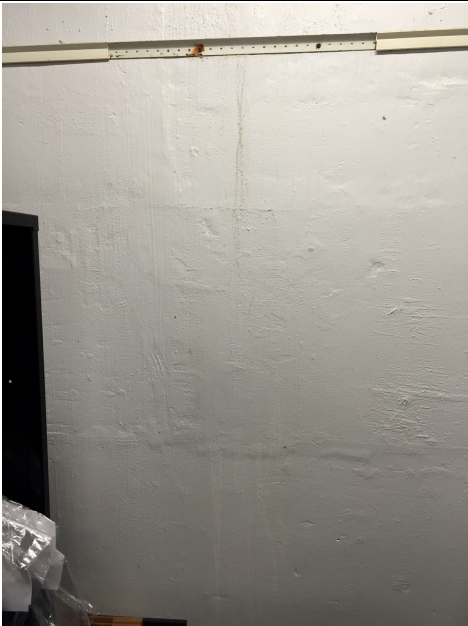
Location 2 – Before repair.
