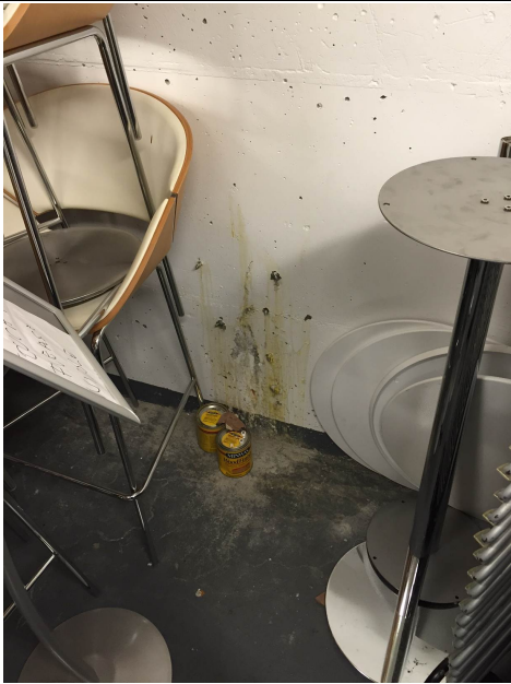
Location 1 – Before repair.
