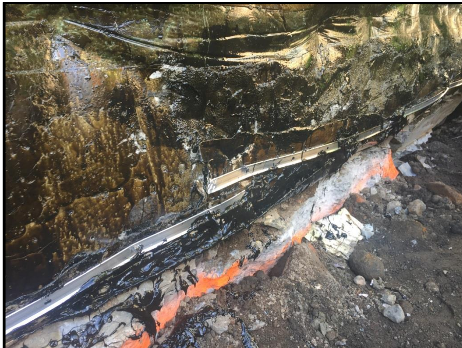
Photo 2: View of Preprufe termination at the bottom of the wall
