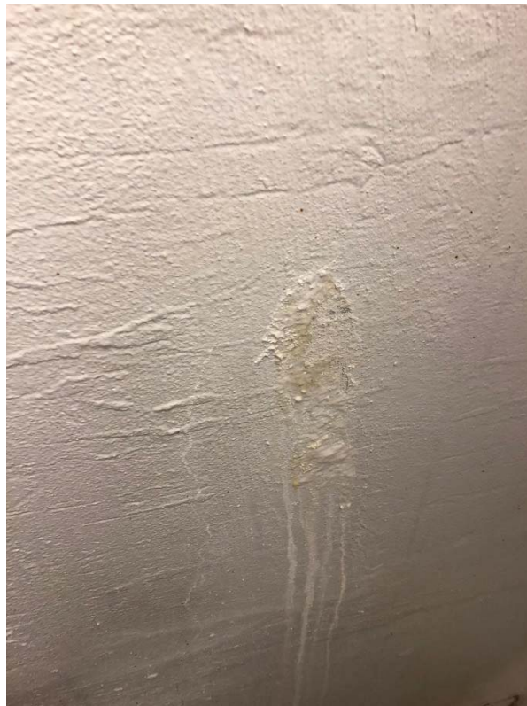
Photograph 4. Water infiltration in northwest basement stairwell (same area as Photo 3, closer picture to show damage detail)
