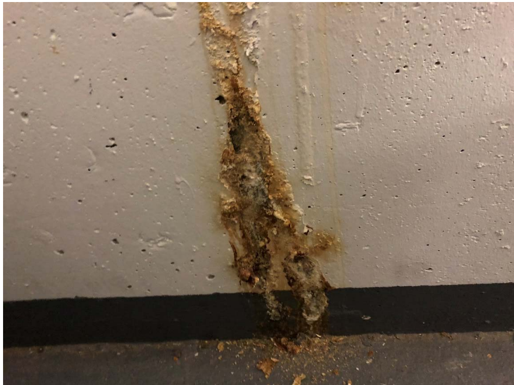
Photograph 2. Water infiltration in Storage Room
