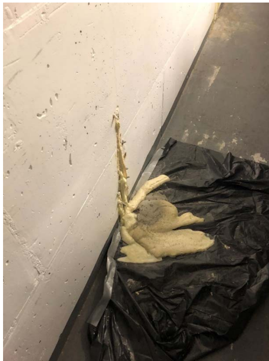
Photograph 4. Injected grout is seeping out of the injection points as it sets (western building perimeter in Storage Room)
