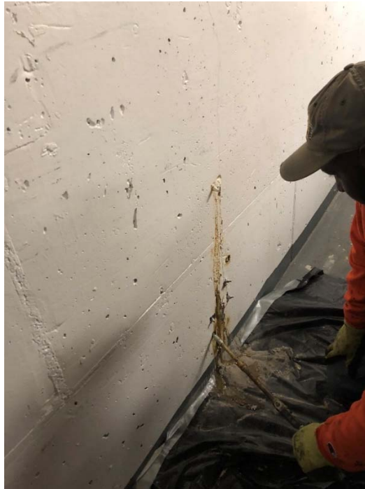
Photograph 3. Contractor injecting grout into points to seal the foundation vapor barrier (western building perimeter in Storage Room)
