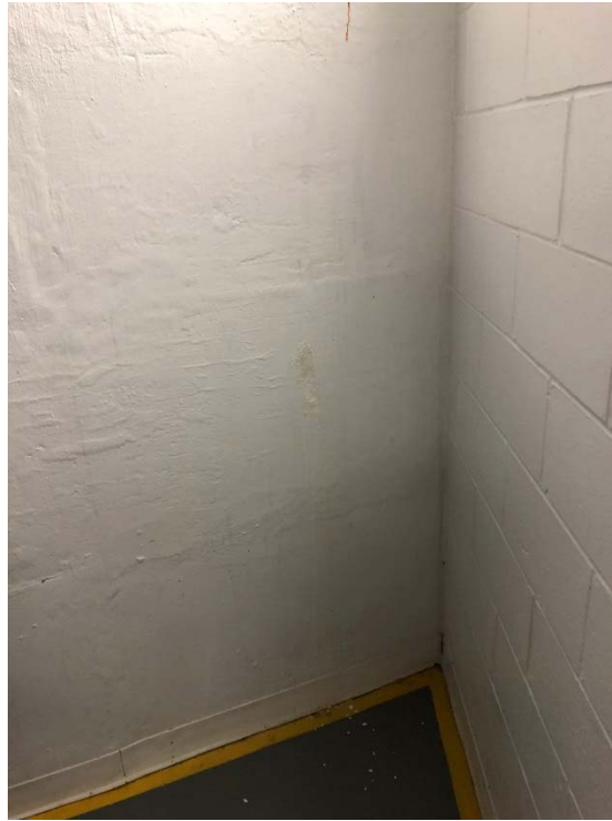
Photograph 3. Water infiltration in northwest basement stairwell
