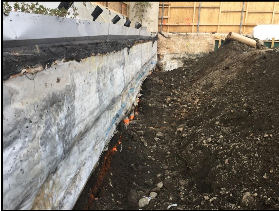
Photo 1: West wall of IAC building prior to beginning waterproofing work (facing northwest)
