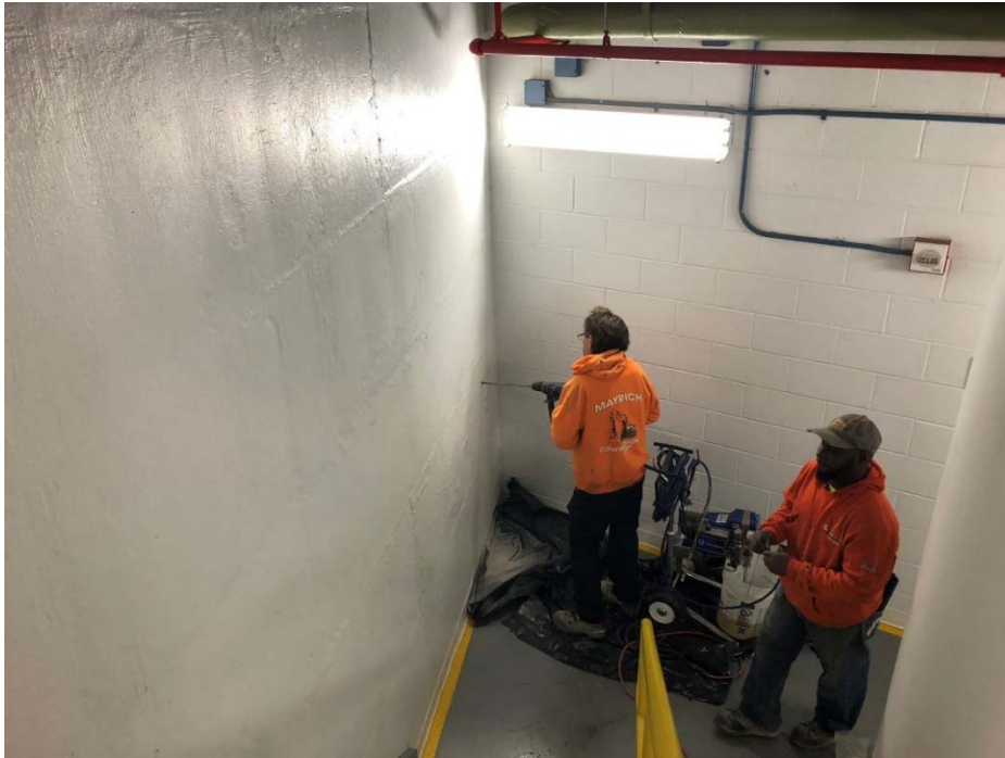
Photograph 1. Contractor drilling holes in the foundation wall for grout injection (northwest corner of building stairwell)
