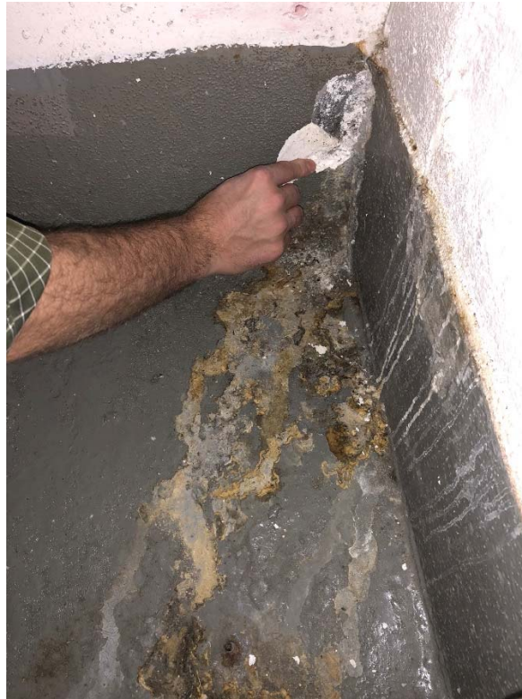
Photograph 1. Water infiltration and dried grout in northeast corner of South Lobby AC Room
