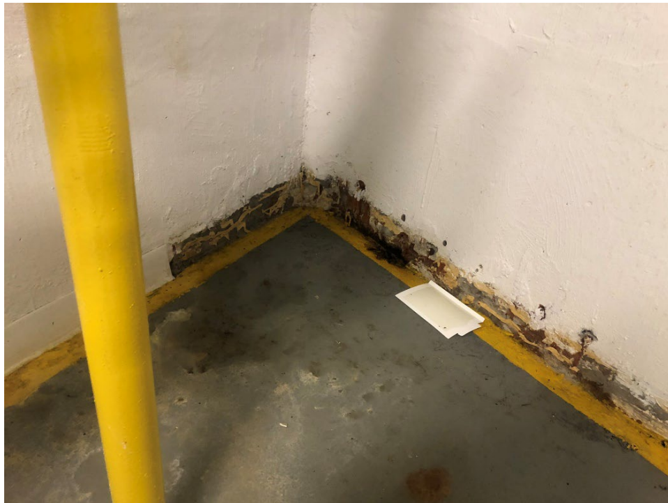
Photograph 2. Corner of Building in North Water Meter Room with Evidence of Water Infiltration (February 9, 2022).
