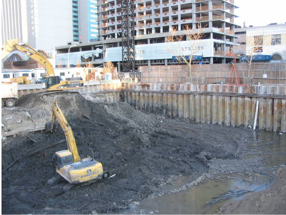
Photograph No. 101: January 26, 2006 – Material load-out operations occurring along western perimeter (view northwest).
