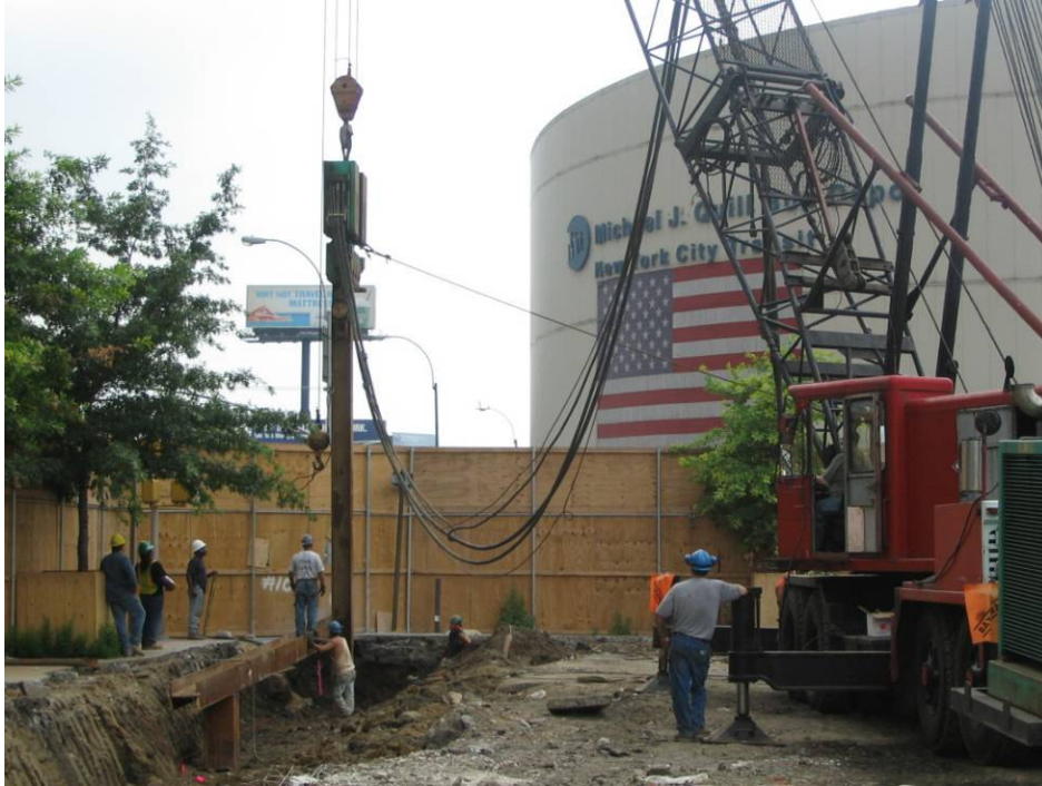
Photograph No. 9: July 15, 2005 - Installing sheet pile section no. 1 in the southeast corner of site.
