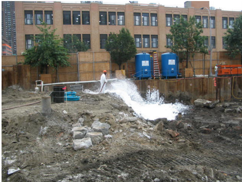
Photograph No. 32: August 31, 2005 - Worker applying foam odor suppressant to area where USTs were discovered and decommissioned (view east).
