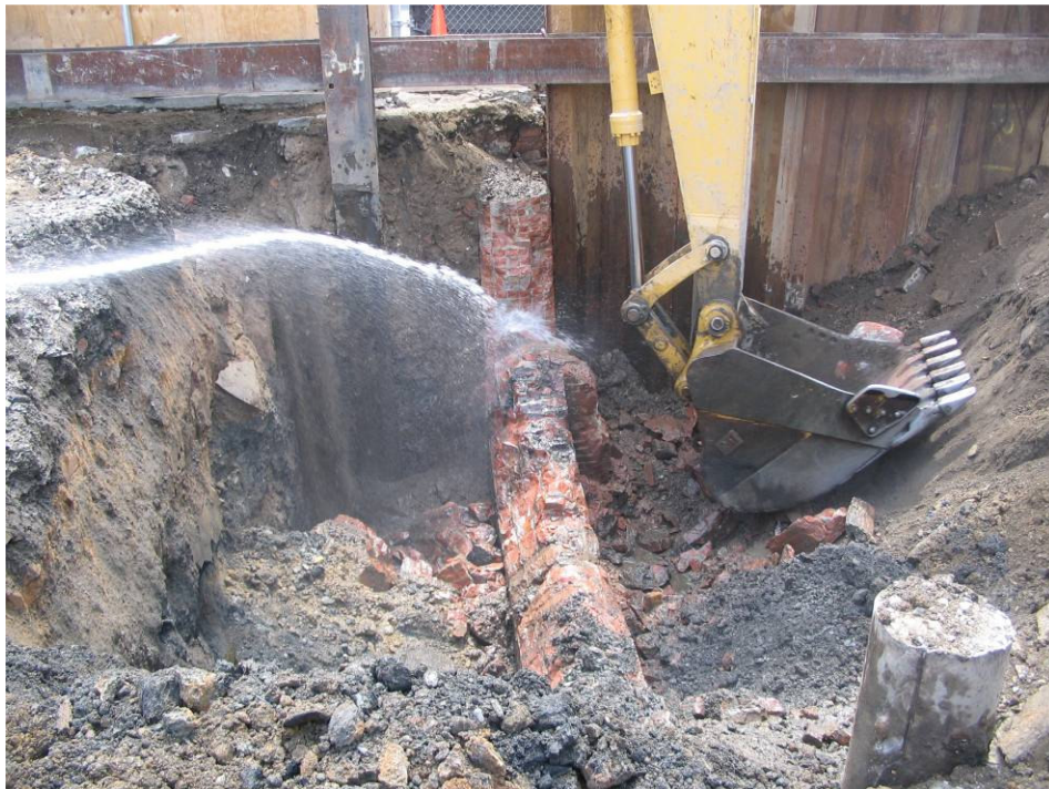
Photograph No. 14: August 6, 2005 - Exposed section of MGP holder wall being excavated and simultaneously wetted down to suppress generation of dust.
