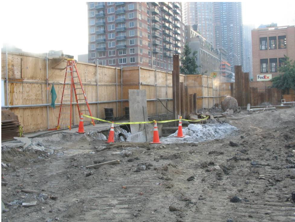
Photograph No. 42: September 13, 2005 - Trench box secured at conclusion of days activities. Note the section of steel plating used to help reinforce the outside edge of the trench box excavation.
