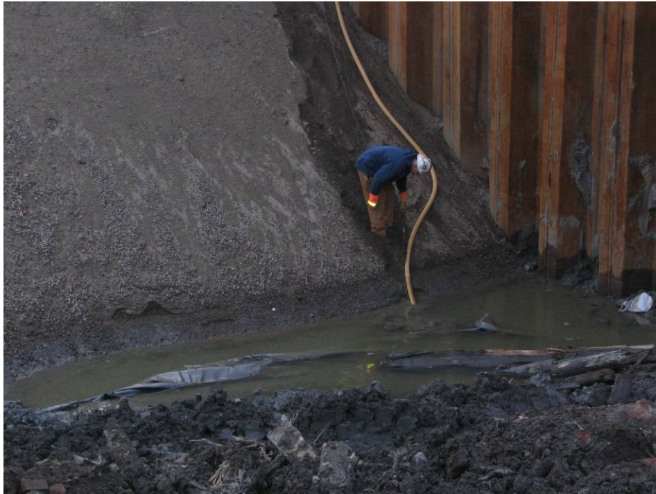
Photograph No. 89: January 10, 2006 - Moretrench worker moving mobile sumps to area with surface water accumulation during dewatering activities.
