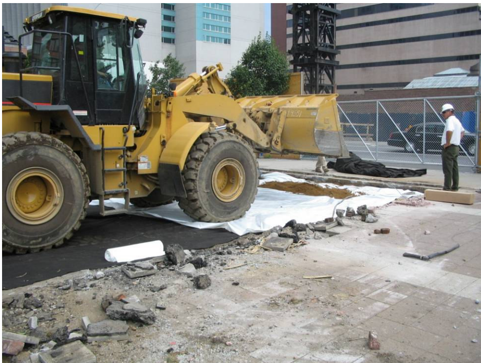
Photograph No. 6: June 2005 - Placing fill material over filter fabric to prepare truck wash area.
