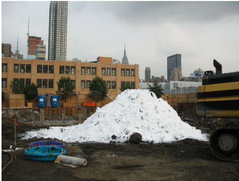
Photograph No. 25: August 2005 - Typical view of foam odor suppressant covering temporary stockpile.
