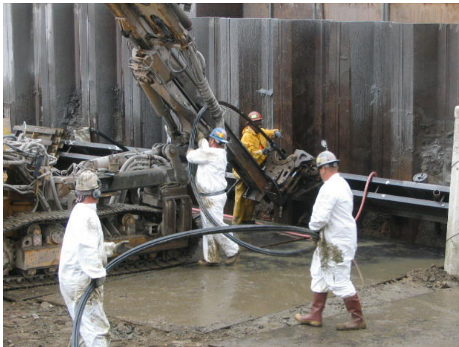
Photograph No. 56: September 29, 2005 - Tie-back anchor tendon being installed into 45-degree angled borehole.
