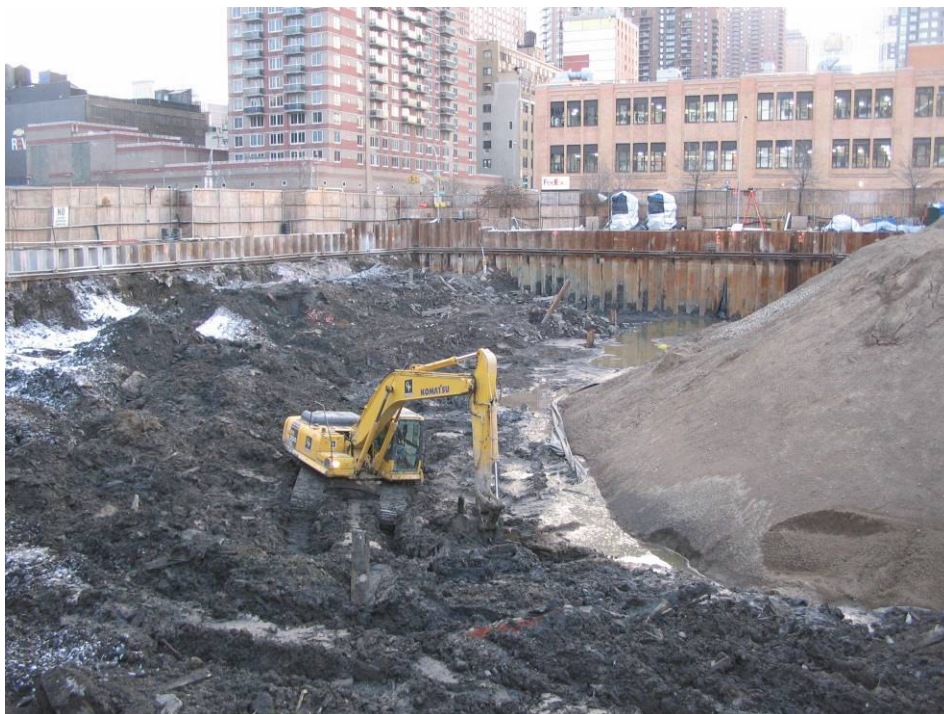
Photograph No. 88: January 10, 2006 - View of excavator working to keep MGP material segregated from RCA stockpile.
