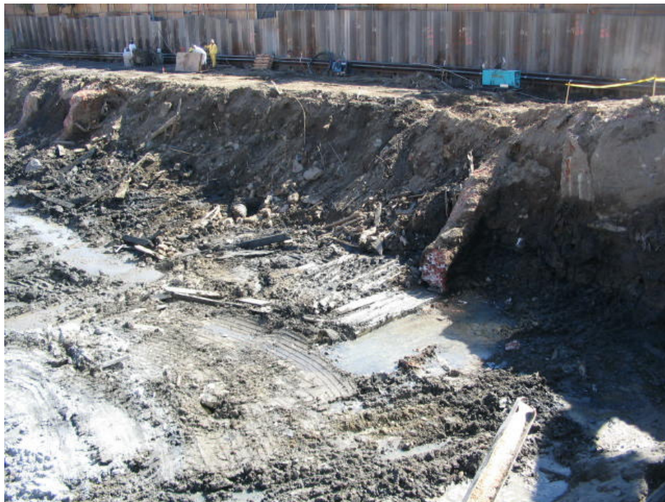
Photograph No. 50: September 21, 2005 - View showing working platform left in place along sheeting wall allowing work to be done on walers in preparation for installation of tie-backs. Note truncated section of MGP holder wall visible within platform.
