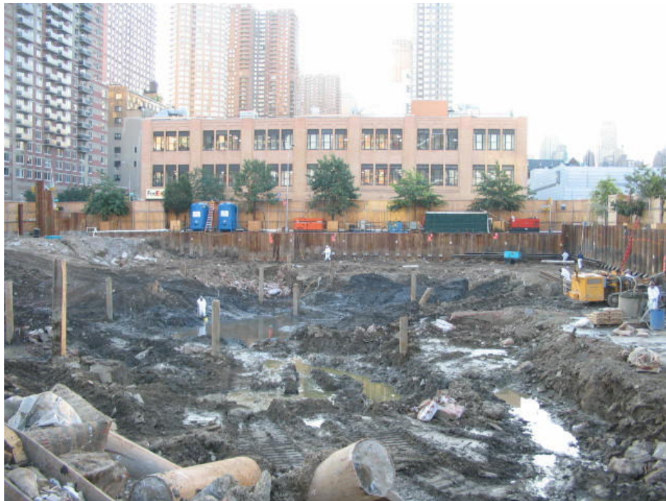
Photograph No. 34: September 2, 2005 - View of excavation (view west). Note position of foam machine along northern site perimeter.
