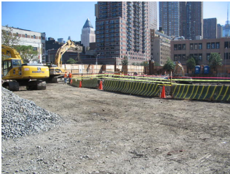
Photograph No. 52: September 22, 2005 - Improved version of work zone demarcation and safety fencing using concrete Jersey barriers and caution tape.
