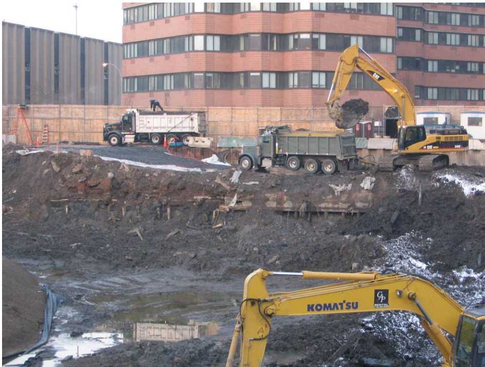
Photograph No. 94: January 13, 2006 - View of material load-out operations (view west). Note remnants of former Purifying House are visible underneath the green truck and excavator and under the inclined roadway leading towards Gate #2.
