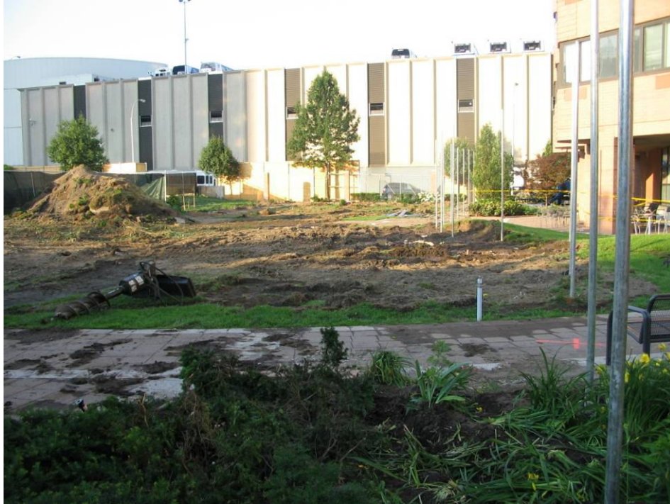
Photograph No. 3: June 2005 - View of park area (view south). Note poles to be used for support of blue perimeter wall.
