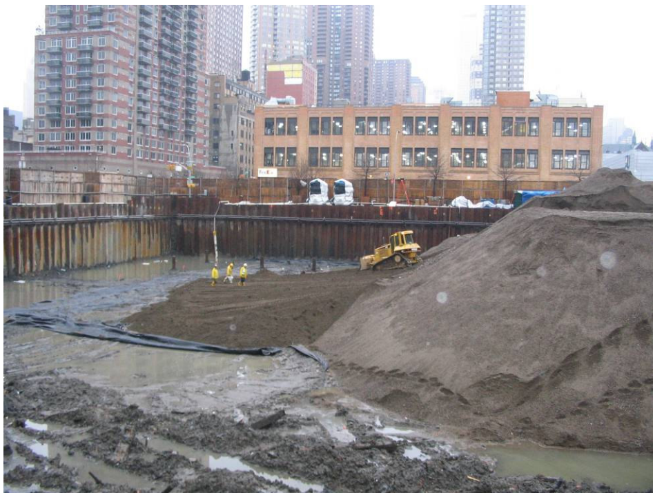
Photograph No. 98: January 23, 2006 – RCA being spread out over emplaced Mirafi 500 geotextile fabric (view northeast).
