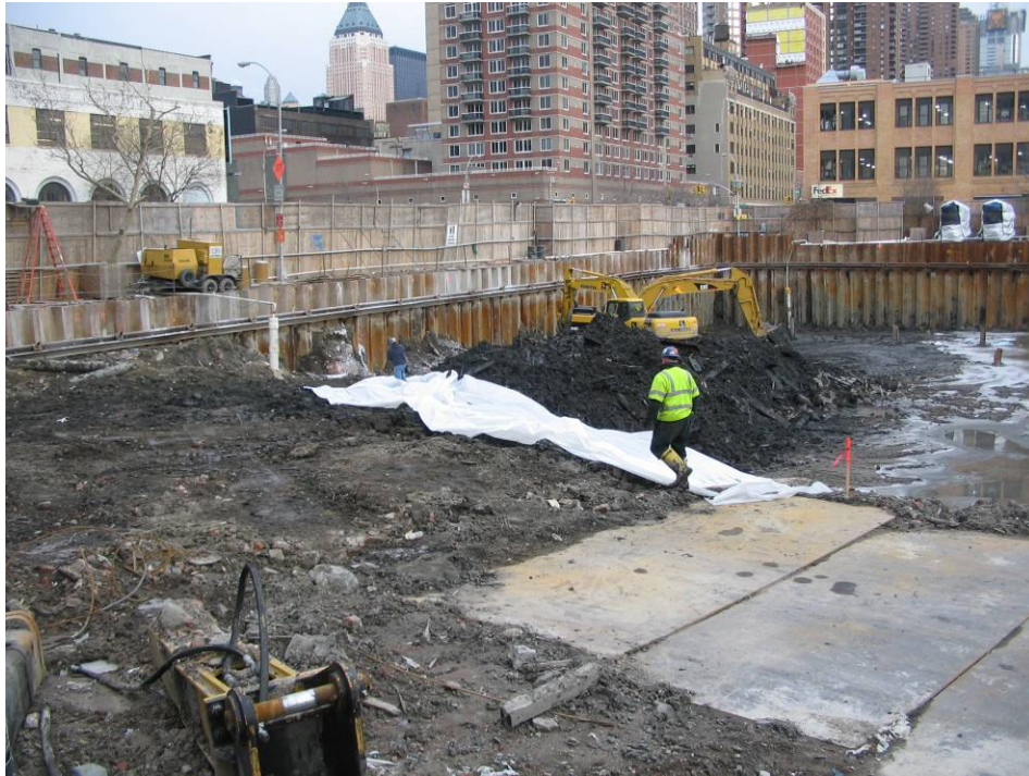
Photograph No. 95: January 17, 2006 – Stockpile being covered with plastic sheeting at conclusion of daily activities.
