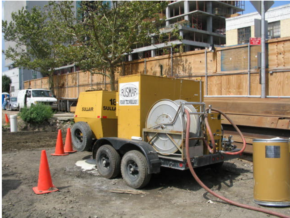
Photograph No. 33: The foam machine.
