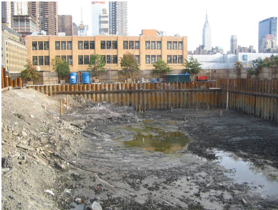
Photograph No. 72: November 1, 2005 - View of excavation looking east. Note that southernmost area of Site has been excavated to depth. Note surface water accumulation present in center of excavation.
