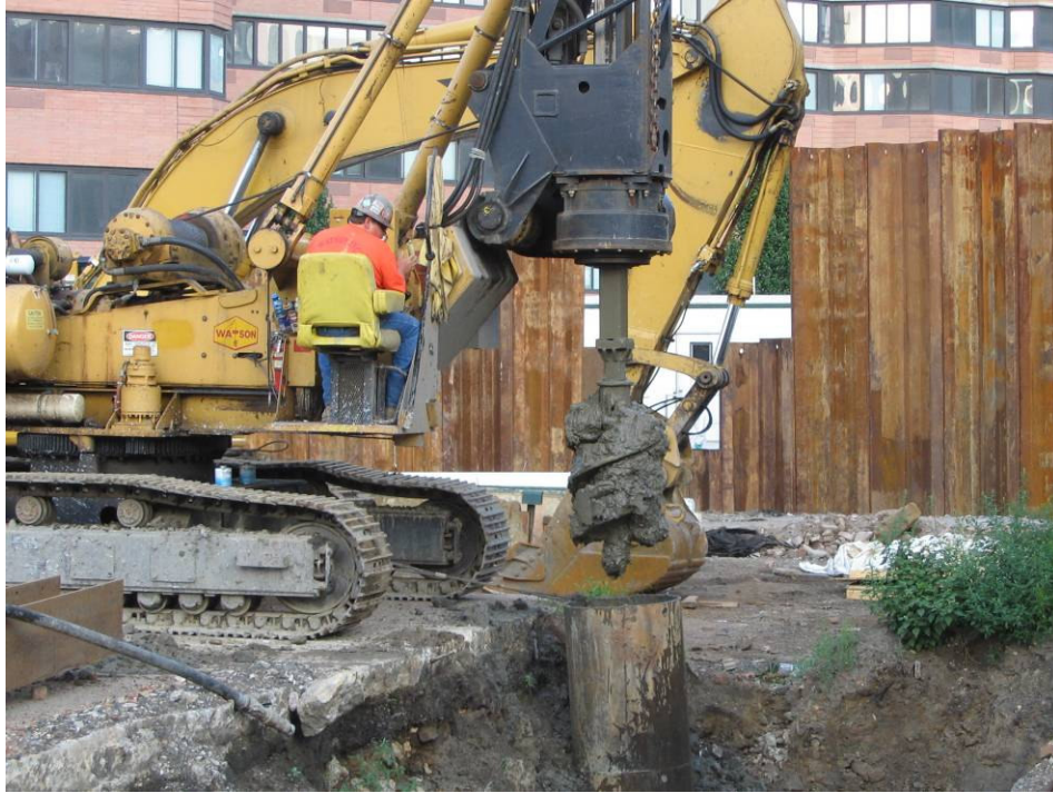
Photograph No. 27: August 18, 2005 - Moretrench's Watson 3-1678 track mounted drill rig advancing borehole for northwestern dewatering well (Well #4).
