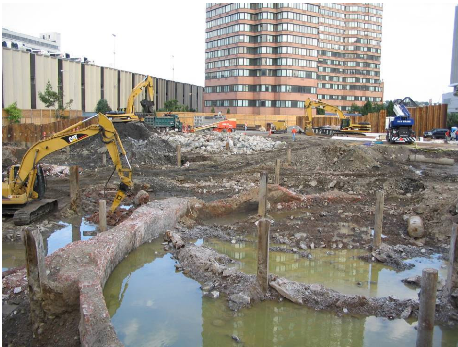
Photograph No. 26: August 18, 2005 - View of excavation showing exposed northeast MGP holder wall, various H-piles and concrete filled pipe piles (view west).
