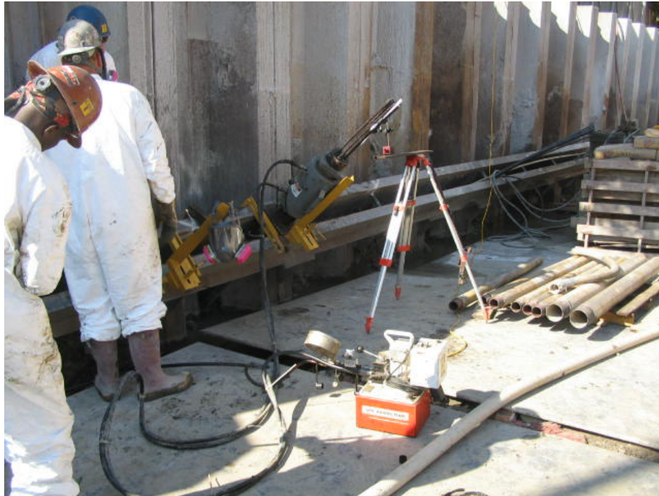
Photograph No. 57: October 3, 2005 - Testing tie-back installation using hydraulic jack and dial indicator to measure elongation.
