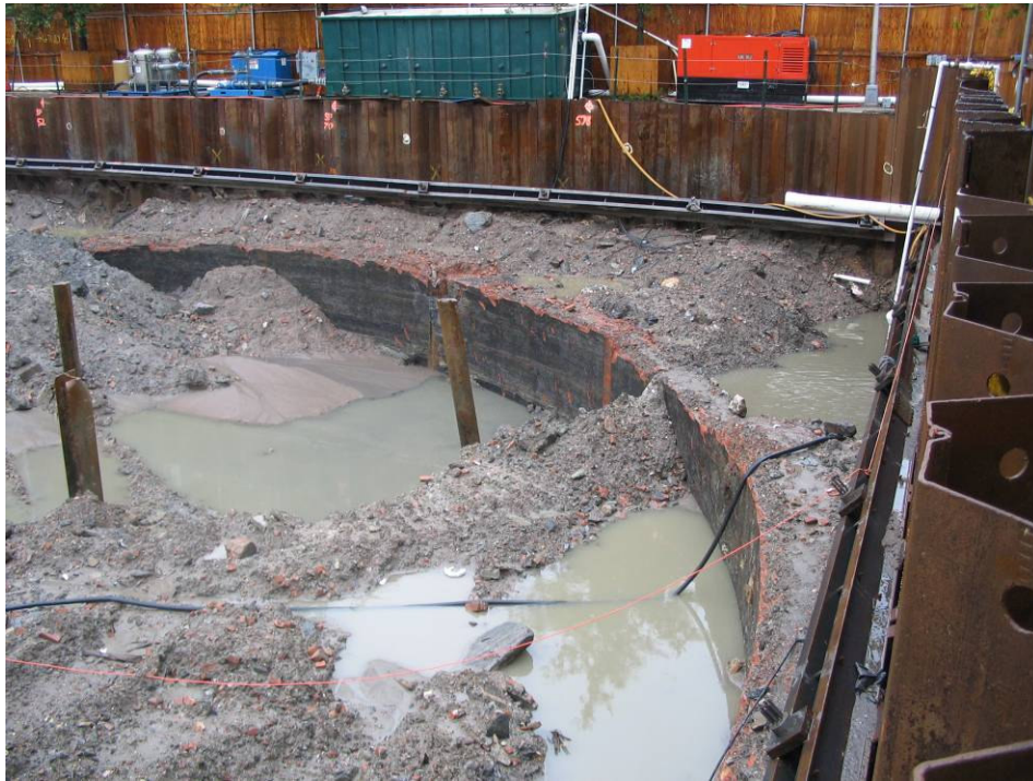
Photograph No. 59: October 14, 2005 - View of surface water accumulation within northeast MGP holder wall remnants. Note presence of hoses and sump pumps used to assist in dewatering efforts.
