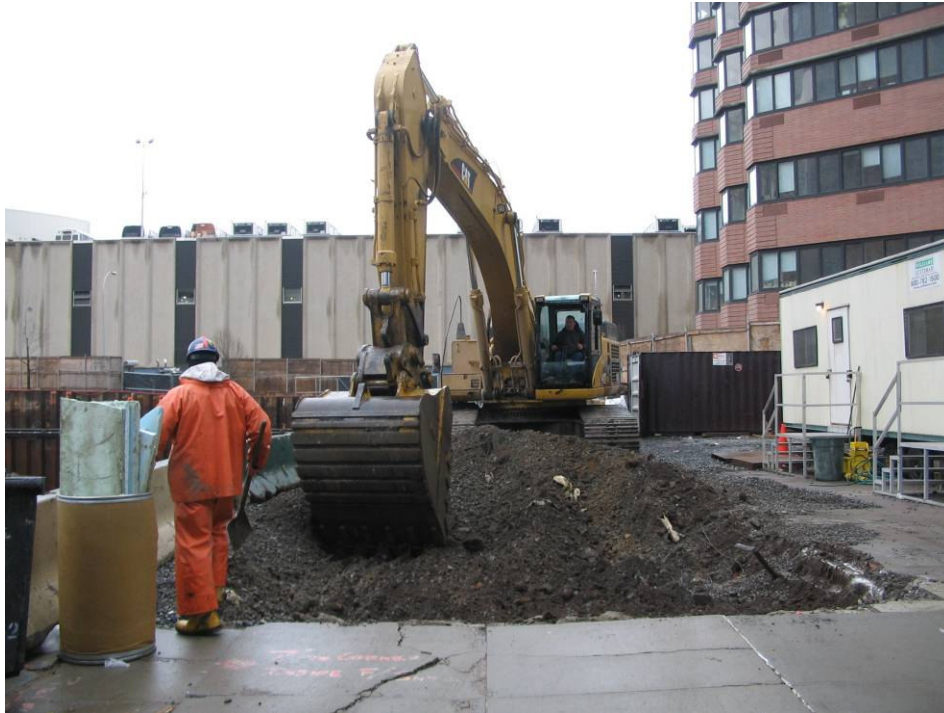
Photograph No. 107: February 3, 2006- Excavator pulling up surface materials in roadway extending from Gate 1 to Gate 2 (view south).
