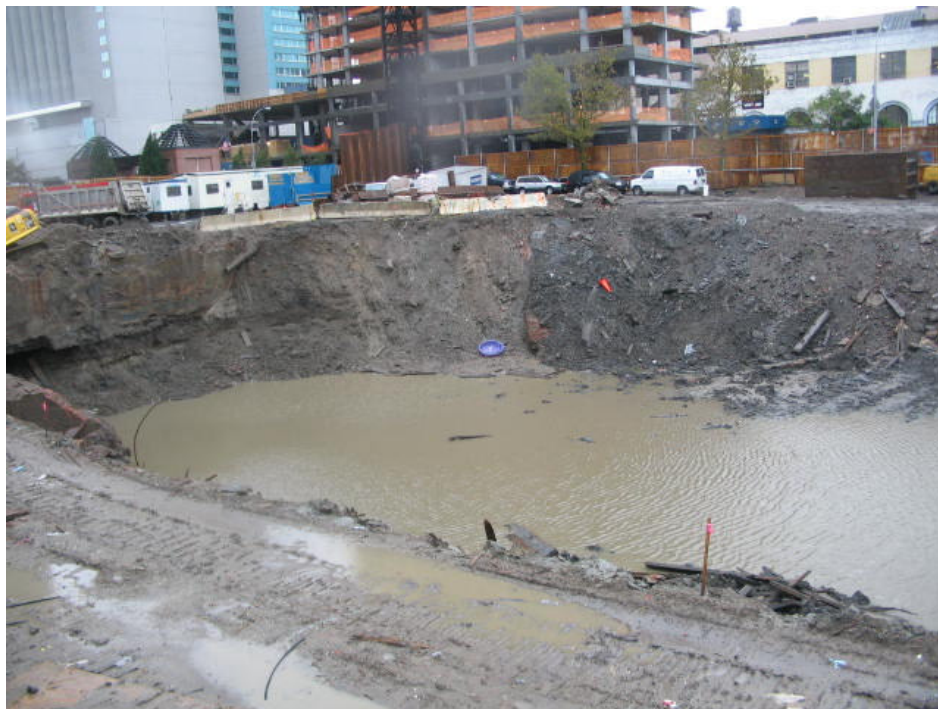
Photograph No. 58: October 12, 2005 - Surface water accumulation from several days of heavy precipitation (view towards northwest).
