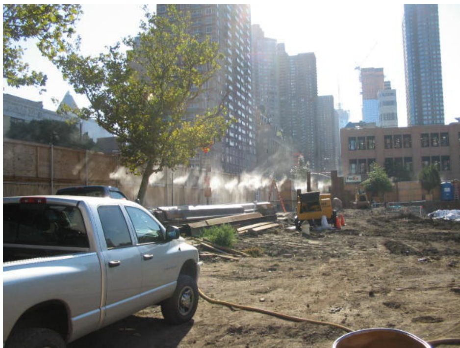
Photograph No. 36: September 6, 2005 - View of Piaan misting system in action (view east along northern perimeter fencing).
