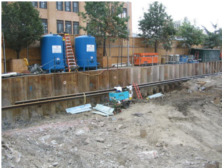
Photograph No. 54: September 26, 2005 - Welders securing walers. Note dewatering treatment system atop eastern sheeting wall.
