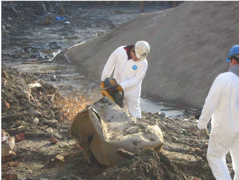
Photograph No. 83: December 9, 2005 - Workers cutting open the UST discovered on 11/18/05 to clean out any residual contents and decommission.
