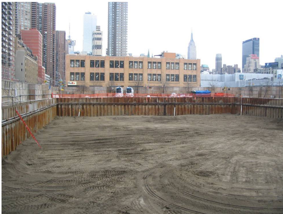
Photograph No. 112: February 9, 2006 – View of Site at conclusion of field activities (view east).
