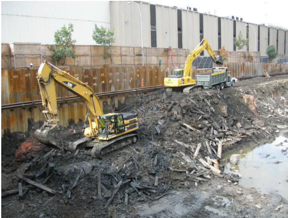
Photograph No. 67: October 25, 2005 - Excavators working in tandem along southern perimeter of Site. Note presence of wood debris (cribbing and planking).
