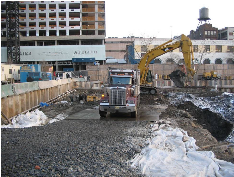
Photograph No. 87: January 10, 2006 - View of reconfigured material load-out area now that trucks are exiting Site via Gate #2 on West 41 st Street (view north). Note steel plates positioned under truck.
