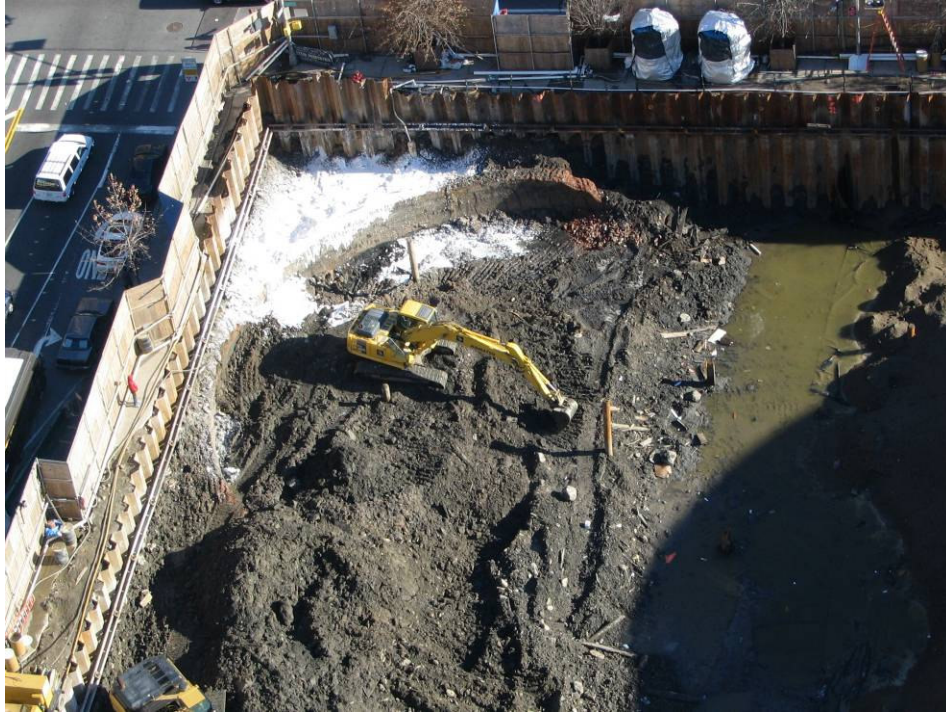
Photograph No. 85: December 30, 2005 - Close-up aerial view of site (view east) from RiverPlace I 32 nd floor observation deck. View is of excavation occurring along northern perimeter now that sheeting installation is complete.
