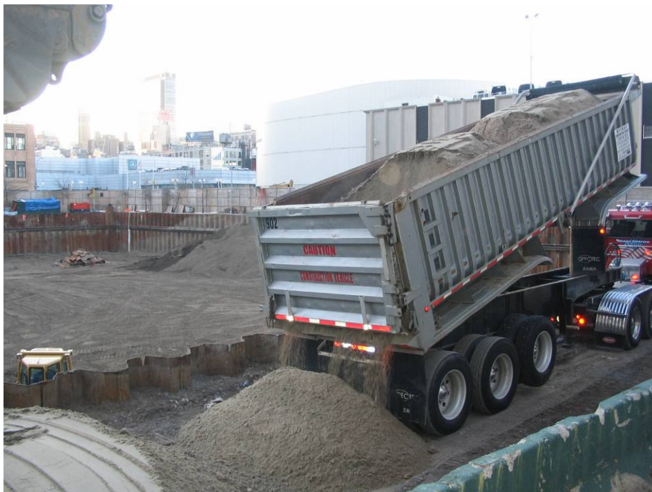
Photograph No. 108: February 9, 2006 – Delivery of imported sand from New York Sand and Stone to infill roadway from Gate 1 to Gate 2 (view southeast).
