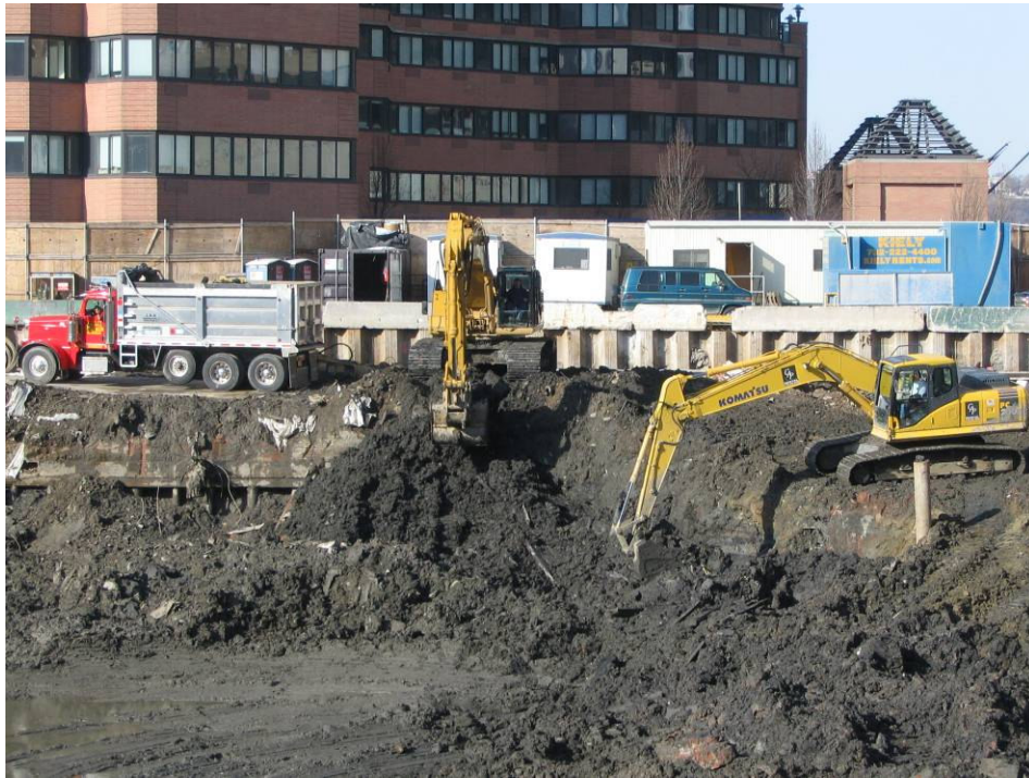
Photograph No. 91: January 12, 2006 - View of excavators working in tandem to load-out material along northern and western perimeter of Site.
