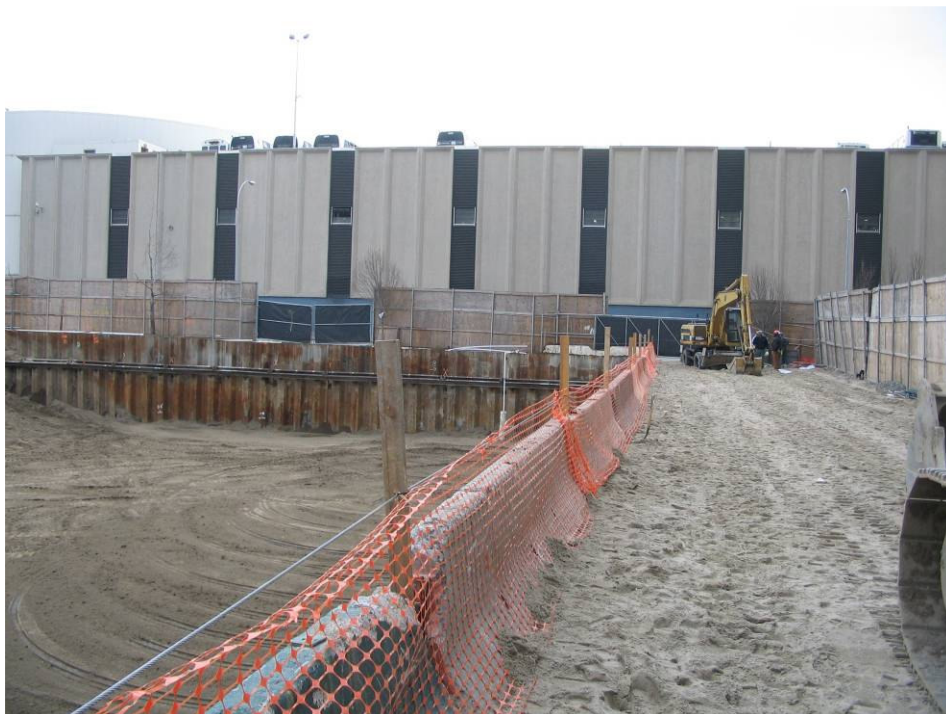
Photograph No. 110: February 10, 2006 – View of roadway between Gate 1 and Gate 2, with fall protection in place, after import of sand from New York Sand and Stone (view south).
