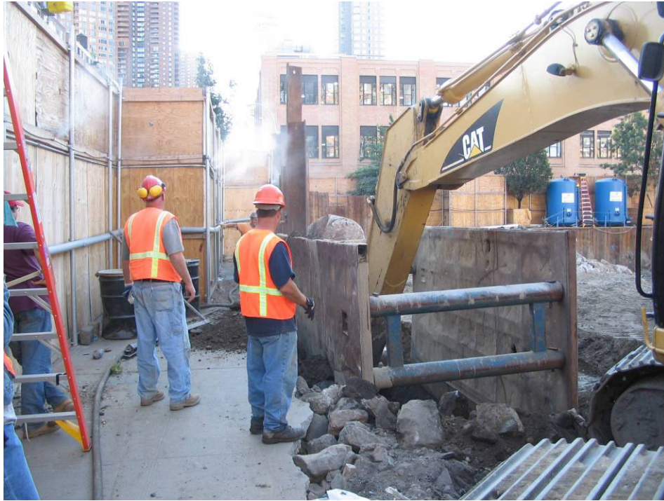
Photograph No. 39: September 10, 2005 - Trench box excavation in progress along northern site perimeter (view east).
