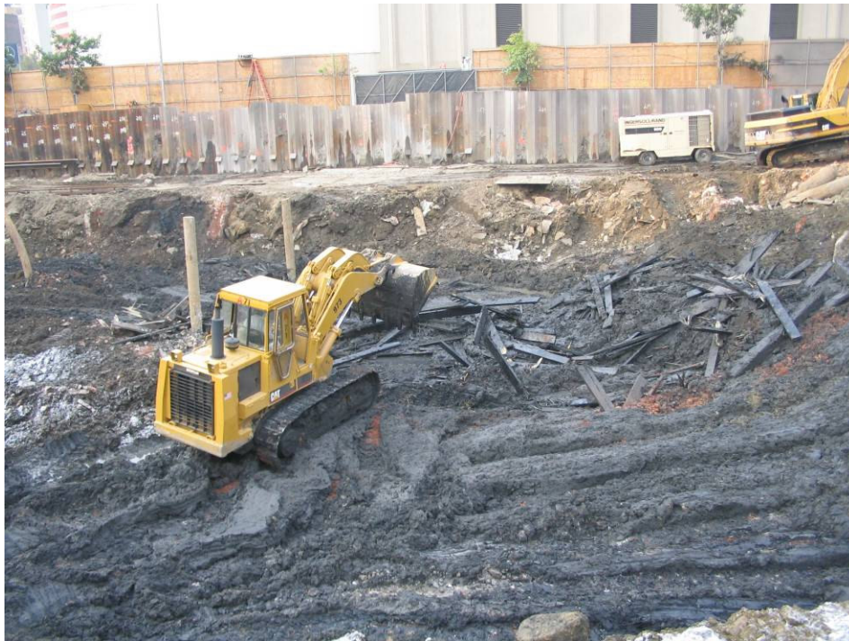
Photograph No. 38: September 9, 2005 - View of wood debris (cribbing and planking) present within excavation (wood present primarily at a depth of approximately 15 to 18 feet below ground surface).
