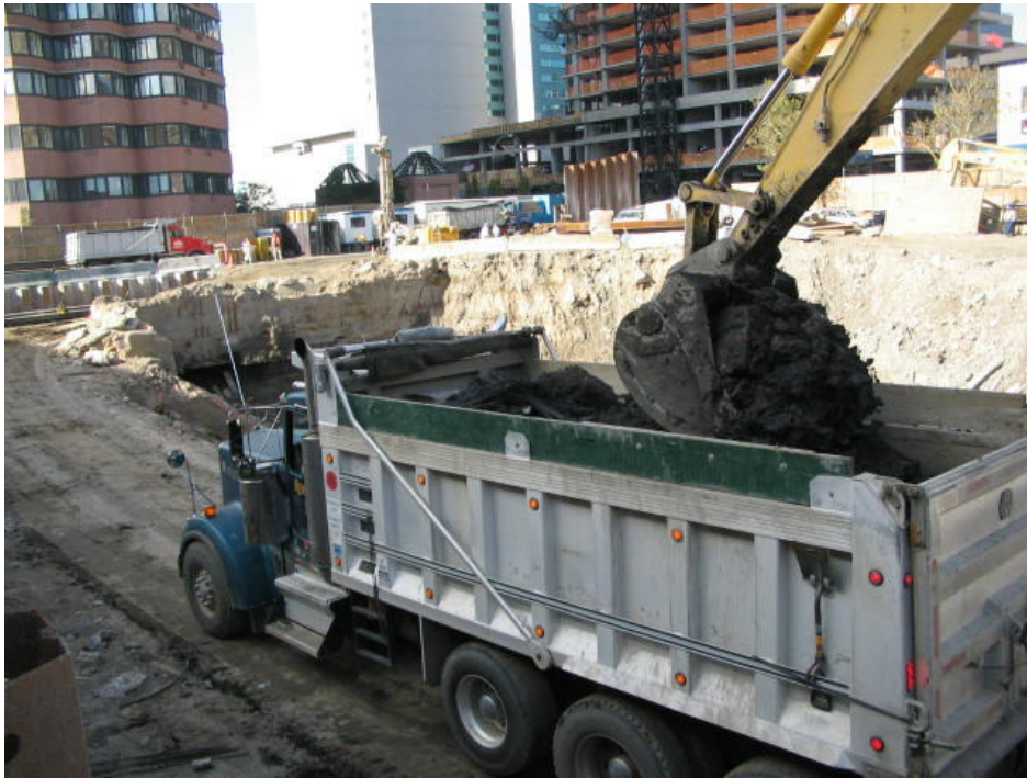
Photograph No. 63: October 20, 2005 - View of material load-out occurring along the southern perimeter of the Site (view towards northwest).
