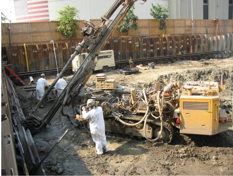
Photograph No. 43: September 13, 2005 - Moretrench drilling 4-inch diameter angled boreholes (45-degree angle) through sheeting for tie-back installation.
