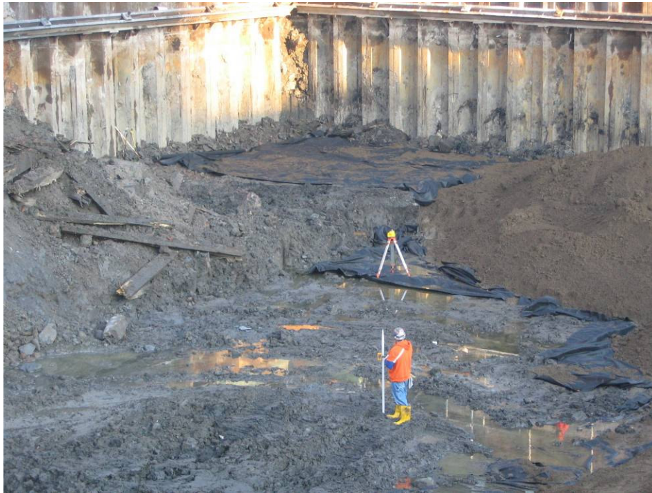
Photograph No. 103: January 30, 2006 – Worker surveying the bottom of excavation before RCA is spread to that area.
