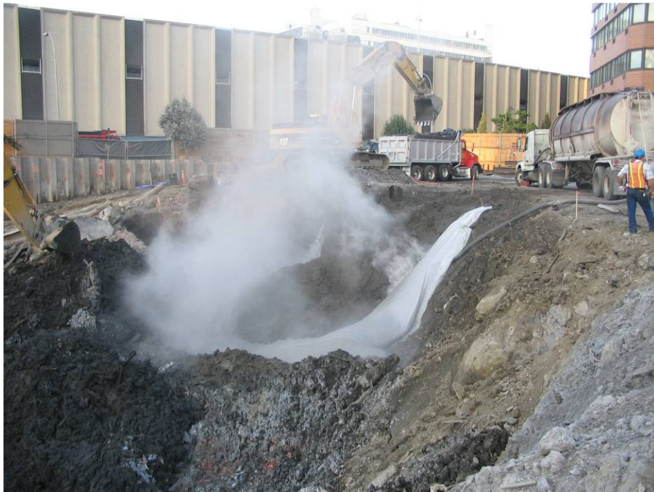
Photograph No. 44: September 14, 2005 - Dust cloud generated during delivery and offloading of Calciment/kiln dust used for stabilization of excavated material.
