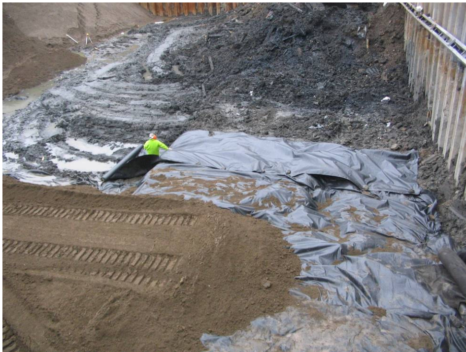
Photograph No. 104: January 31, 2006 – Worker emplacing Mirafi 500 geotextile fabric atop the westernmost portion of the excavation. Note that this portion of the Site was excavated to approximately el -8.5 (remainder of Site excavated to el -13).
