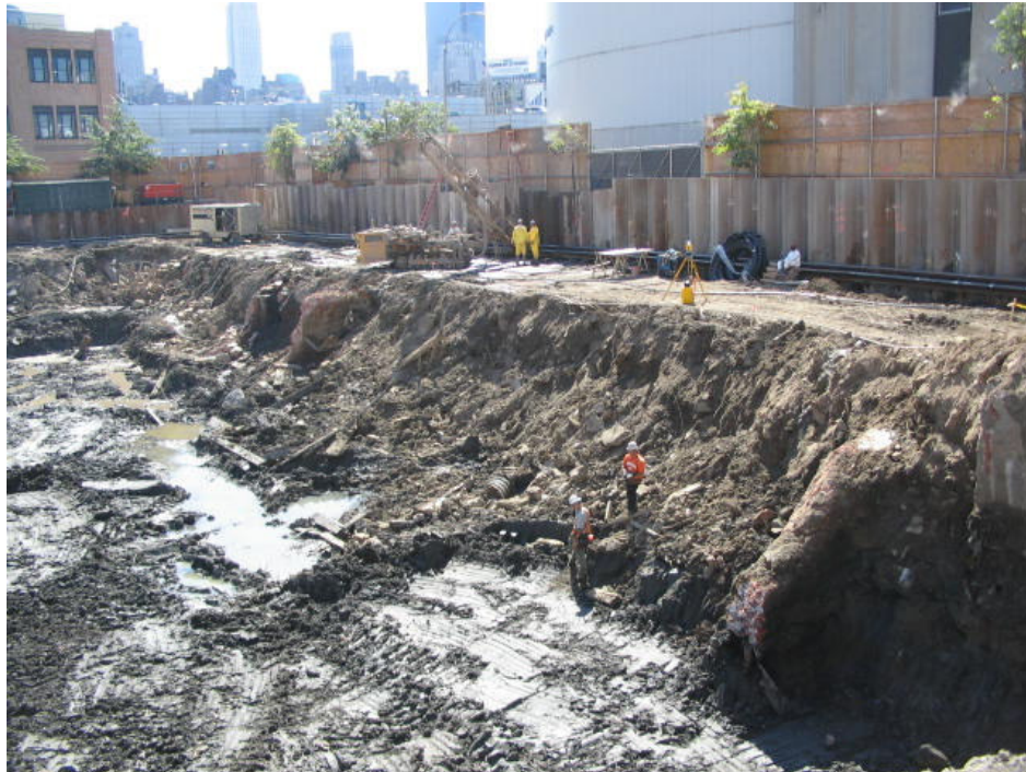
Photograph No. 51: September 22, 2005 - Another view of working platform temporarily left in place along sheeting line (view towards southeast).
