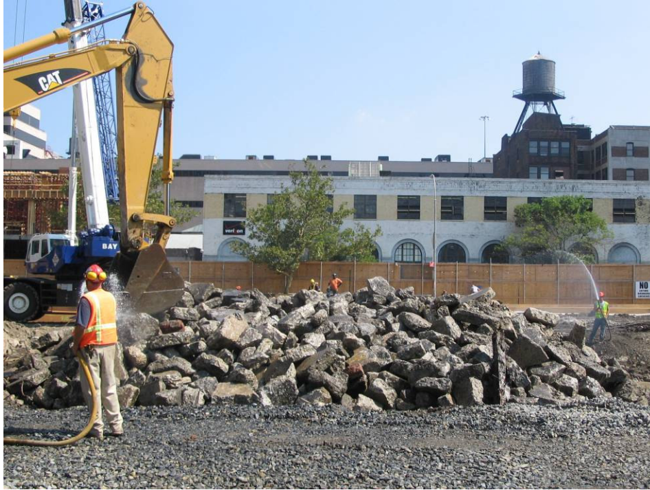
Photograph No. 11: August 2005 - Stockpile of C&D material being wetted down to minimize generation of dust.
