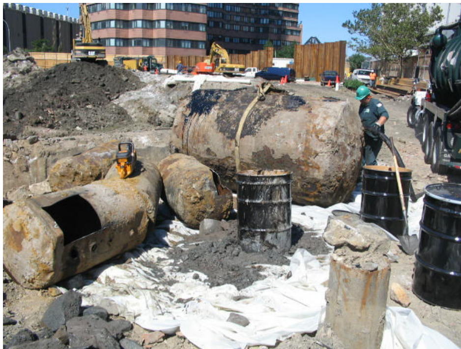
Photograph No. 28: August 25, 2005 – Additional USTs discovered in northeast portion of Site having contents vacuumed out and cleaned for decommissioning.
