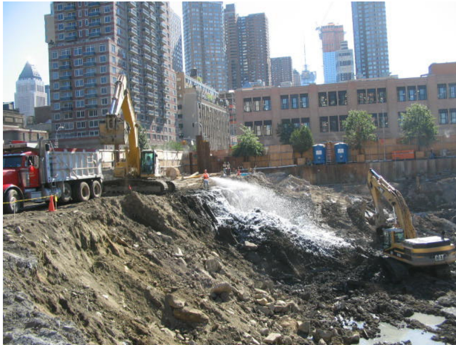
Photograph No. 49: September 21, 2005 - Workers keeping area covered with foam during excavation activities.
