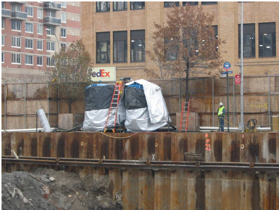
Photograph No. 82: November 28, 2005 - View of dewatering treatment system carbon vessels prepped for winter with insulated jackets.
