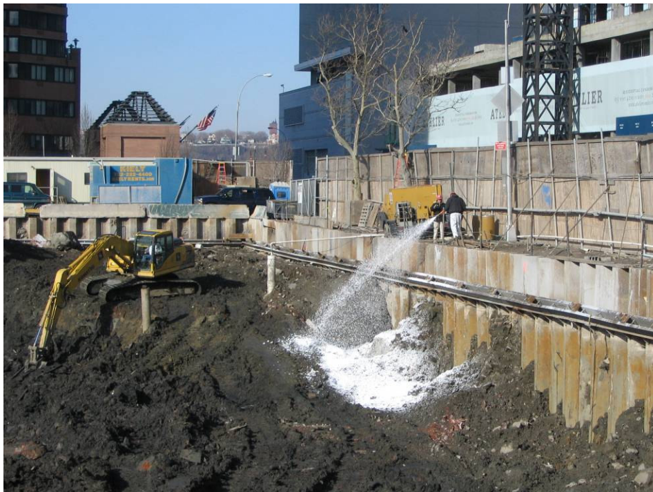
Photograph No. 92: January 12, 2006 - Foam being applied as excavator works in northwestern corner of Site.
