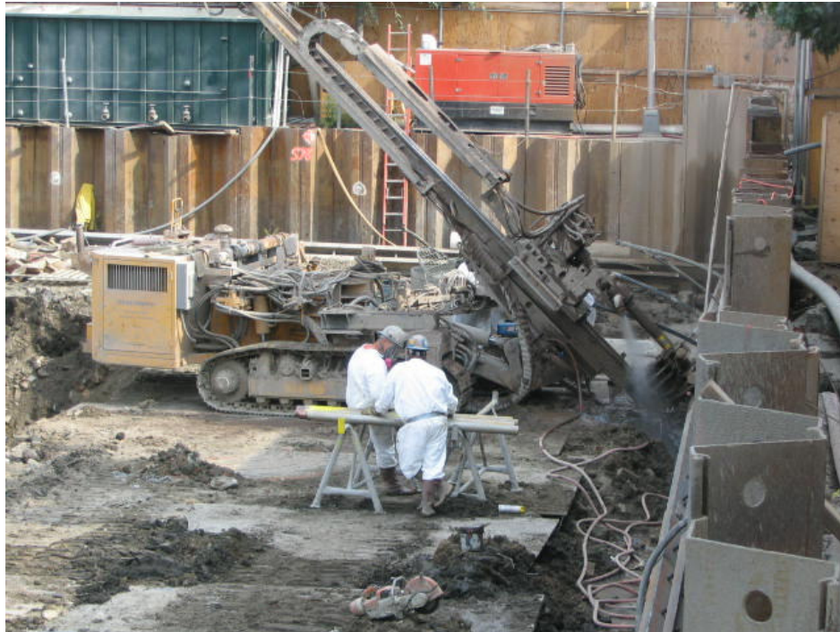
Photograph No. 47: September 19, 2005 - View showing angled boring for tie-back installation in progress.
