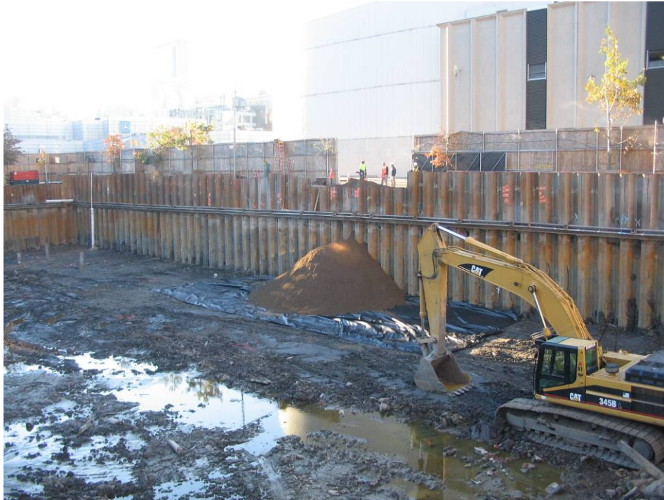
Photograph No. 75: November 7, 2005 - View of first load of imported RCA material atop section of Mirafi 500 geotextile fabric. RCA delivered through Gate #4.
