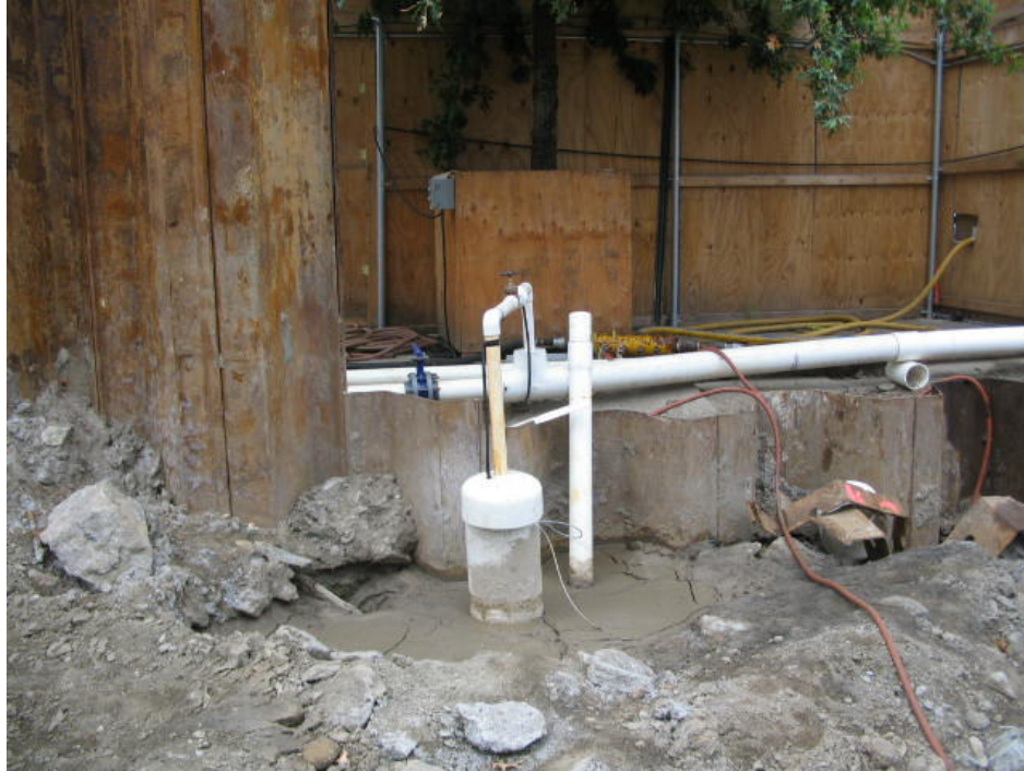
Photograph No. 31: August 2005 - Typical view of dewatering well assemblage.
