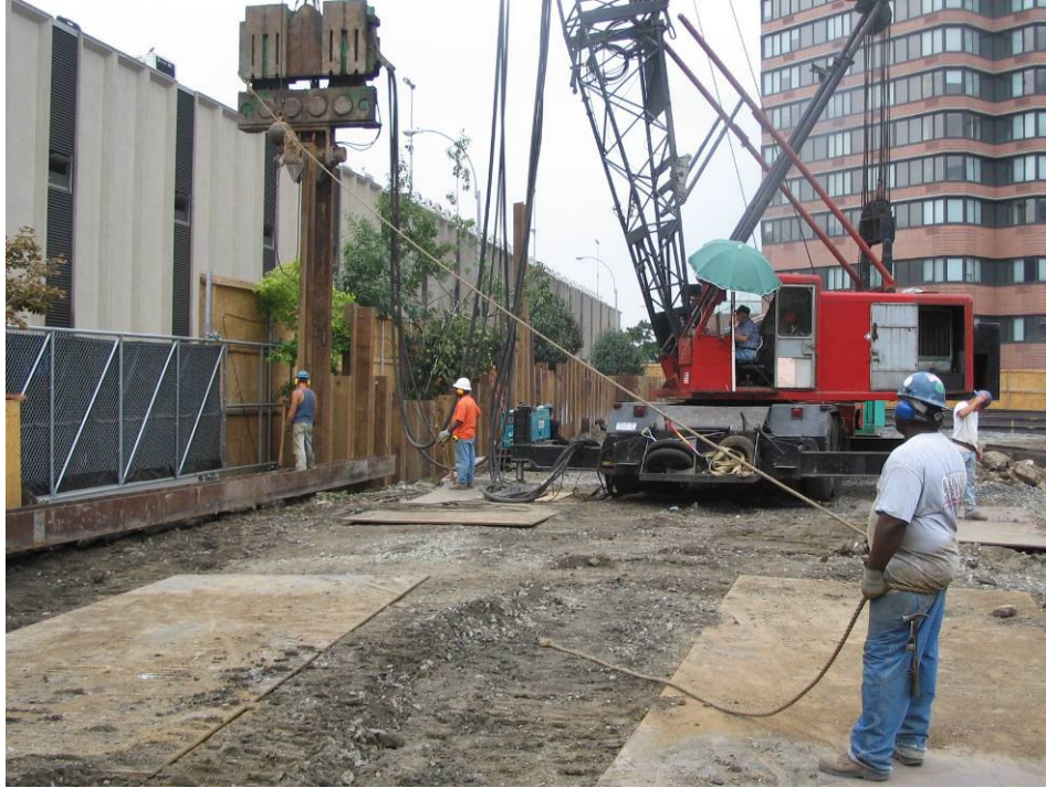
Photograph No. 15: August 9, 2005 - Sheet piling installation occurring in southwest corner of Site and proceeding towards the east.
