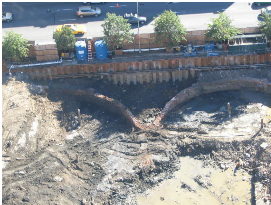
Photograph No. 62: October 19, 2005 - Aerial view zoomed into to highlight the exposed section of the northeast and southeast MGP holder walls.
