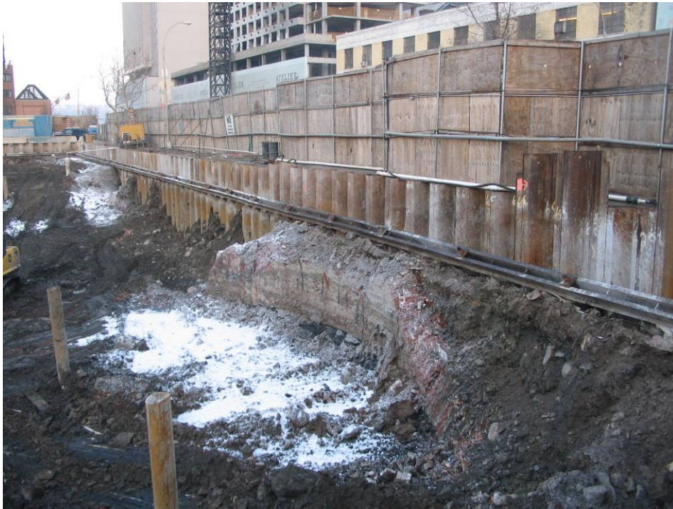
Photograph No. 93: January 13, 2006 - View of remnant of northeast MGP holder wall (view towards northwest).
