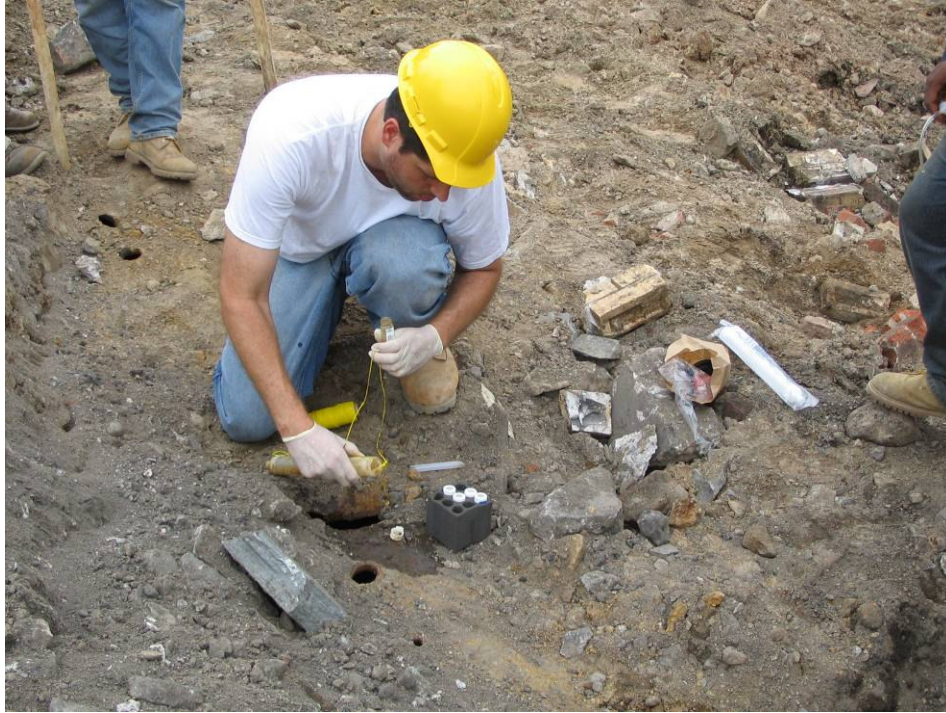
Photograph No. 17: August 9, 2005 - Collecting sample of contents from UST discovered in northeast portion of Site.
