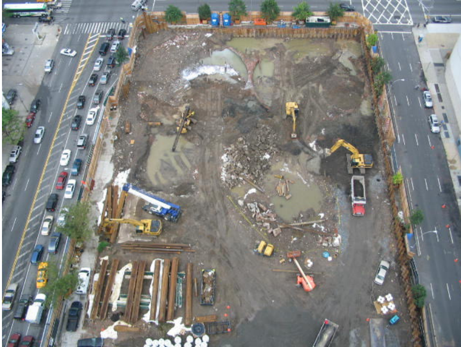
Photograph No. 21: August 15, 2005 - Aerial view of site (view east) from RiverPlace I 32 nd floor observation deck. Note the tops of the northeast and southeast MGP holder walls are visible where the two holders are conjoined.
