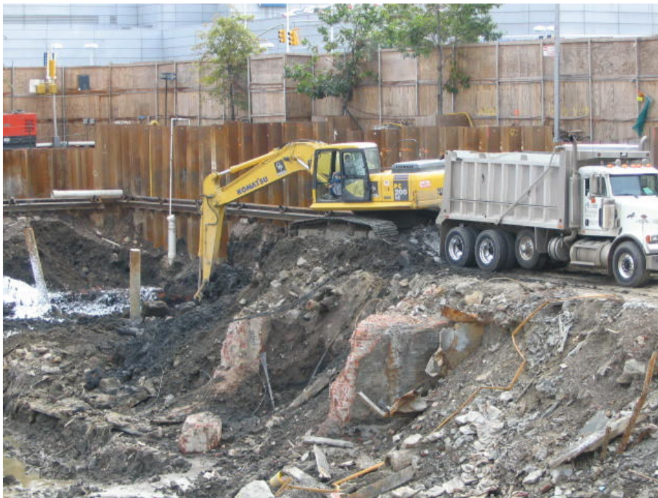
Photograph No. 64: October 20, 2005 - Material load-out occurring along southern perimeter of Site (view towards southeast). Note southeast dewatering well in background of photo (Well #2).
