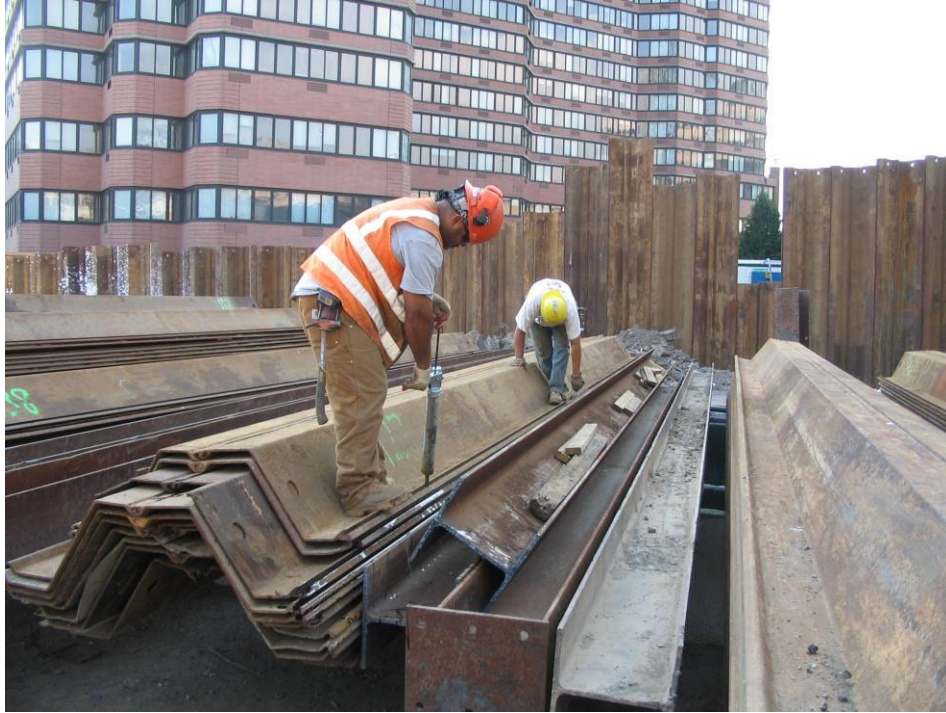
Photograph No. 13: August 2005 - Preparing sheeting sections with Adeka Ultra Seal A-50 waterproof sealant.
