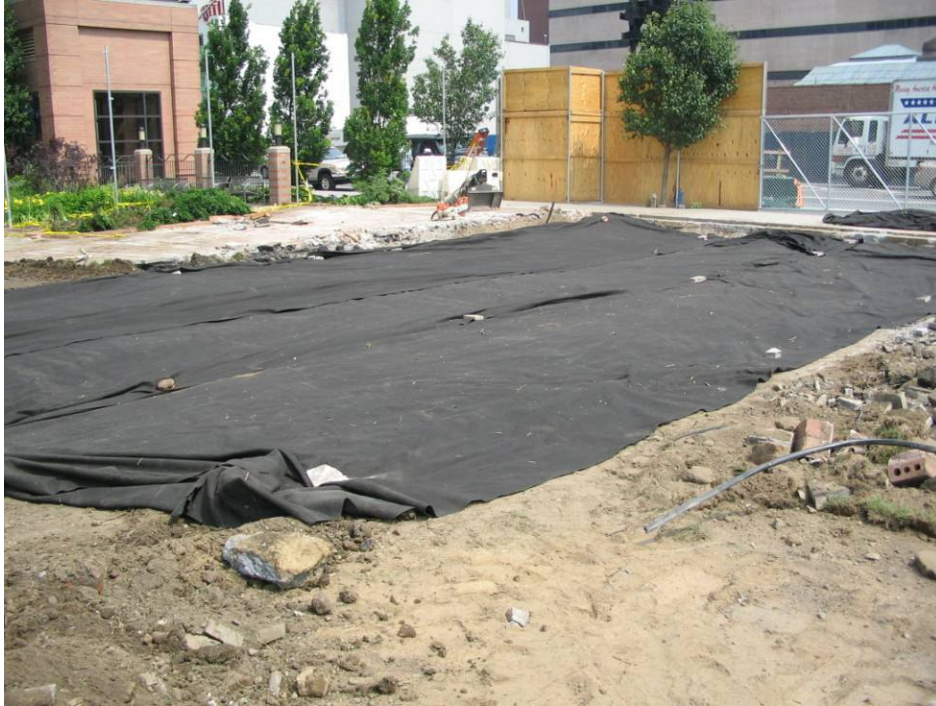
Photograph No. 5: June 2005 - Filter fabric emplaced in front of Gate #1 (view towards northwest).
