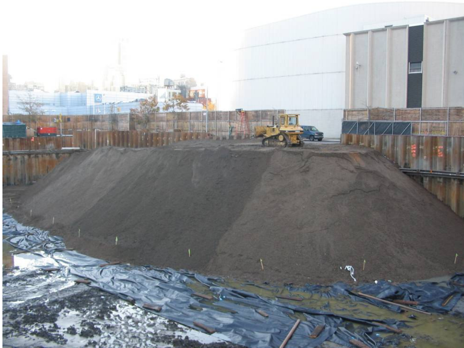
Photograph No. 81: November 17, 2005 - View of RCA stockpile before beginning to spread material across extent of excavation.
