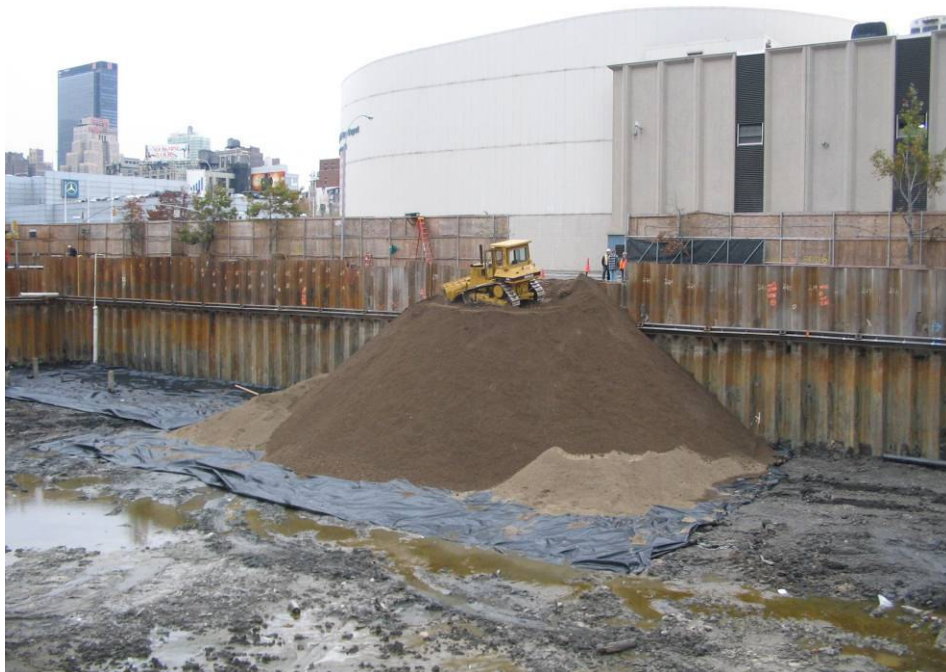
Photograph No. 76: November 9, 2005 - Continued stockpiling of RCA material. Bulldozer on top of stockpile was used to spread out the RCA material.
