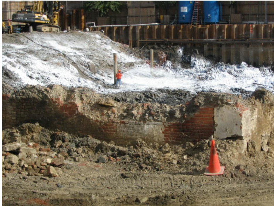
Photograph No. 65: October 20, 2005 - View showing exposed former MGP-related structure (view towards northeast). Note foam odor suppressant covering area.
