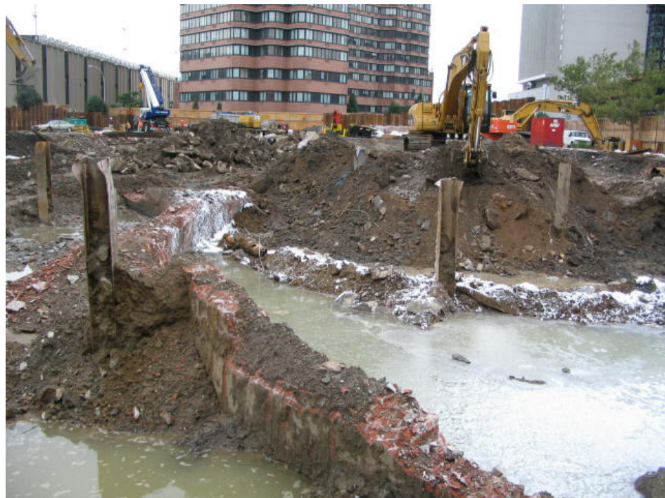
Photograph No. 20: August 15, 2005 - View of exposed section of northeast MGP holder wall (view west). Note surface water accumulation and/or exposed groundwater.
