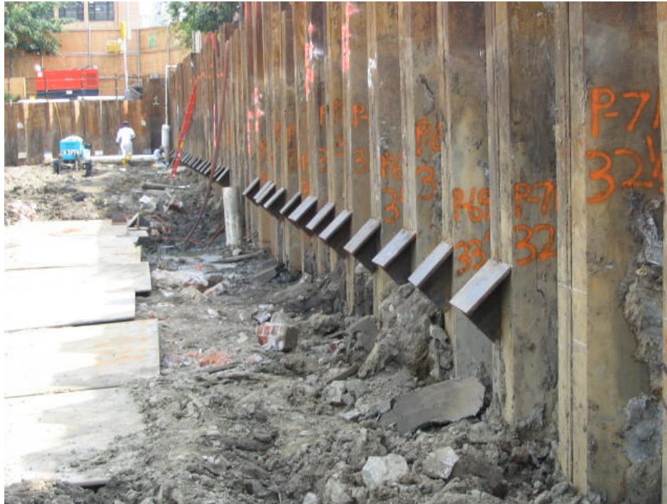
Photograph No. 29: August 29, 2005 - View of seats for waler installation along southern sheeting line (view east).
