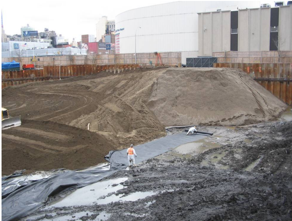
Photograph No. 99: January 25, 2006 – Workers spreading Mirafi 500 geotextile fabric over bottom of excavation (view south-southeast).
