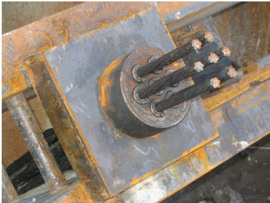
Photograph No. 60: Close-up view of tie-back locked off and set in place with exposed terminus cut to length.
