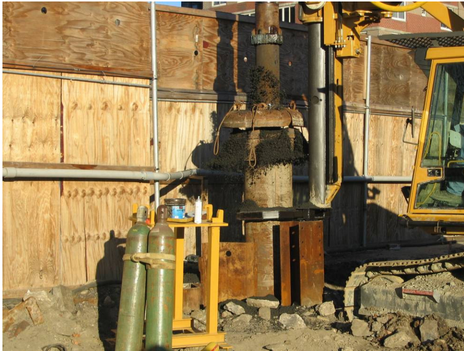
Photograph No. 73: November 2, 2005 - Close-up view of Skanska/Underpinning drill rig clearing subsurface obstacles to facilitate sheeting installation along the northern perimeter. Note cuttings being deflected downwards by shield on drill casing.
