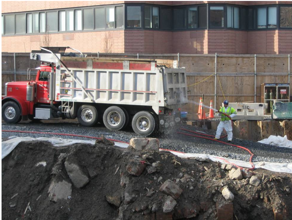
Photograph No. 97: January 20, 2006 – View of alternate truck wash down operation occurring on stone haul road (trucks are exiting onto West 41 st Street).
