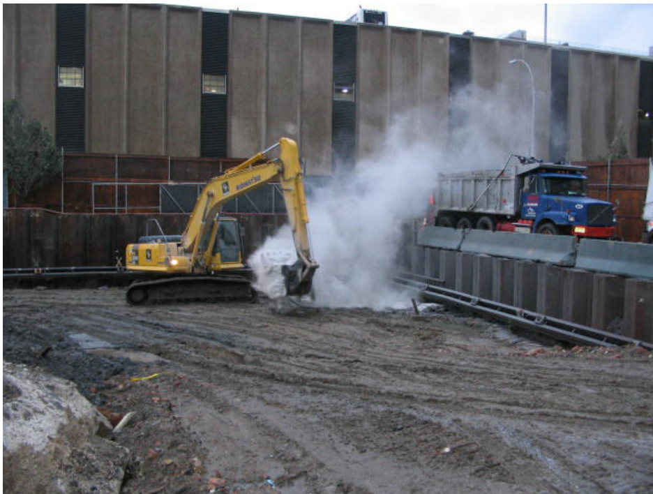
Photograph No. 68: October 25, 2005 - Typical dust generated by excavator gathering scoop of Calciment/kiln dust for material stabilization.
