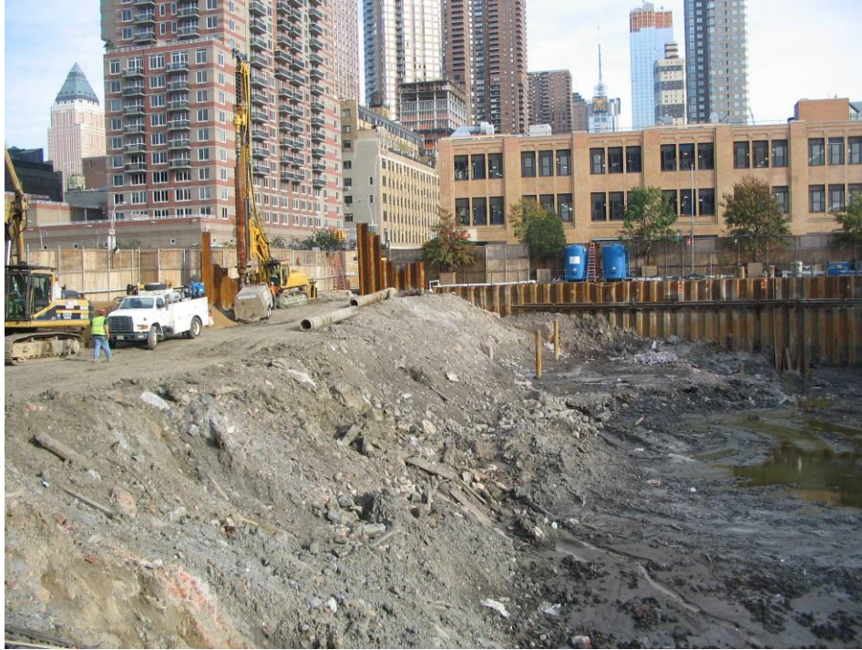
Photograph No. 71: November 1, 2005 - View of excavation looking northeast. Skanska/Underpinning drill rig can be seen clearing subsurface obstructions along northern perimeter.
