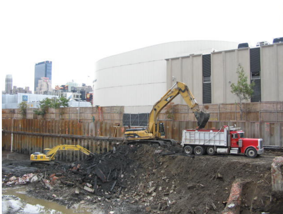
Photograph No. 69: October 27, 2005 - Another view of material load-out operations occurring along southern perimeter of Site. Note how working platform has been removed progressing towards the west.
