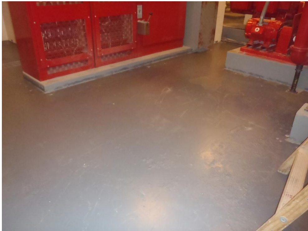
Photograph No. 6: View of cellar floor in the pump room of River Place II.
