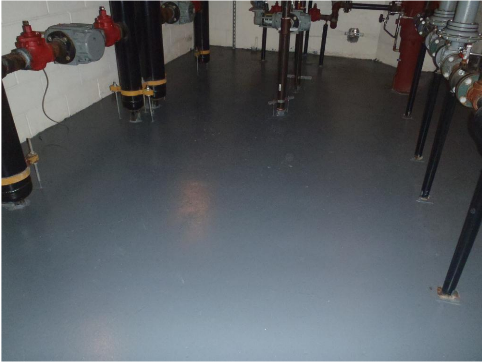
Photograph No. 13: View of concrete floor in lowest level of River Place I.
