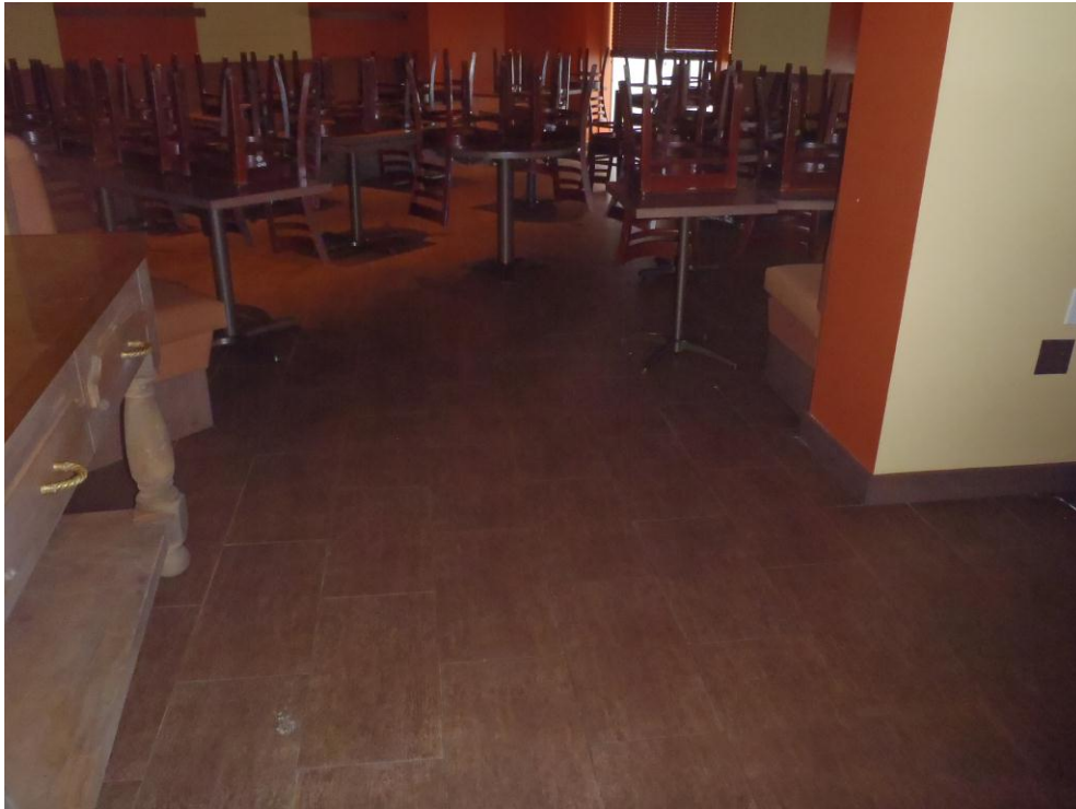
Photograph No. 15: View of surface cover inside restaurant on ground floor of River Place I.
