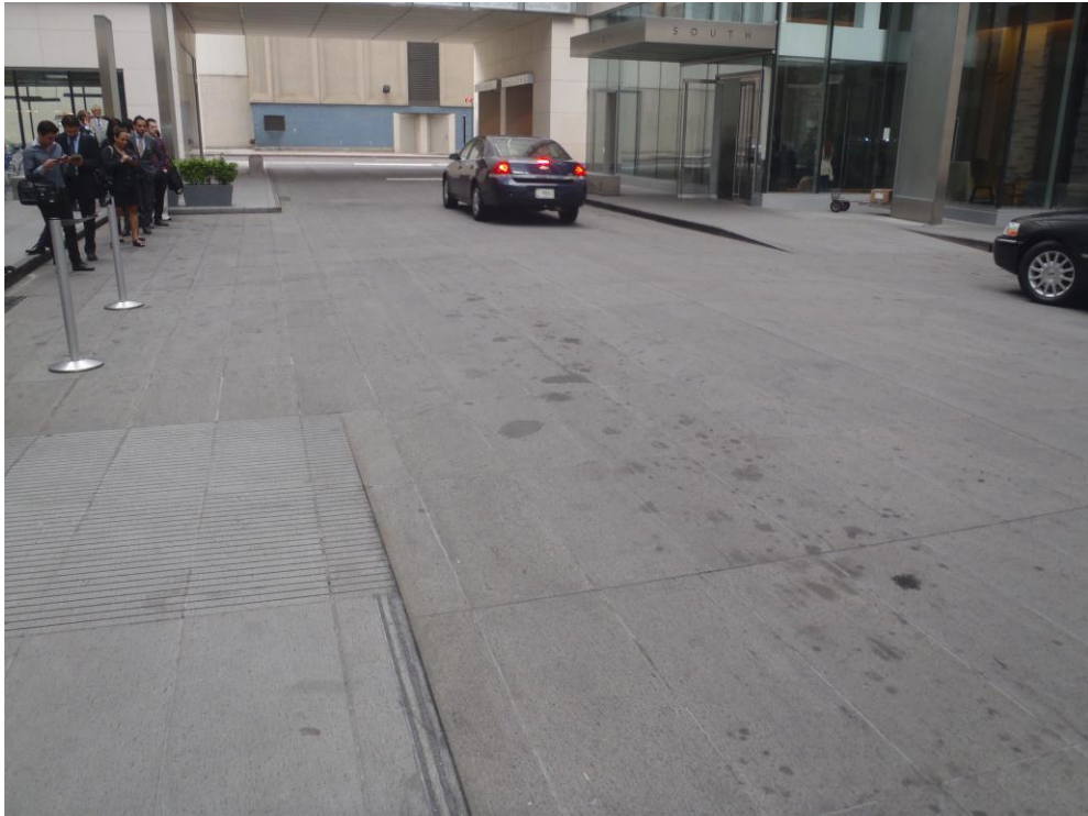
Photograph No. 1: View of paved walkway/driveway area located between River Place II buildings (North and South Towers).
