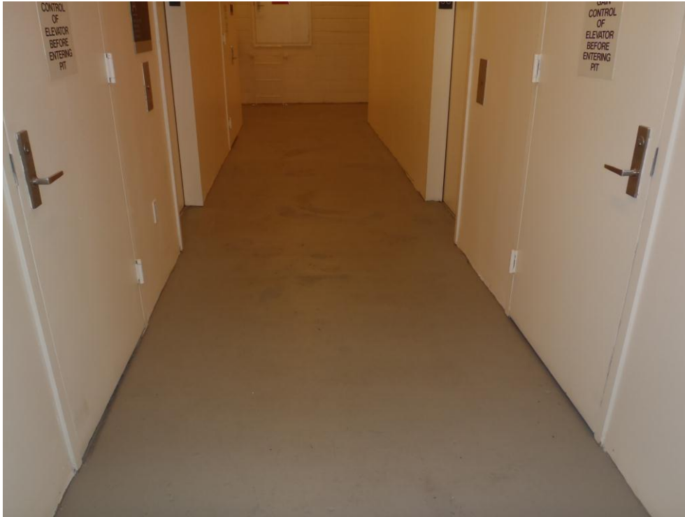
Photograph No. 3: View of hallway floor in lower level of River Place II.
