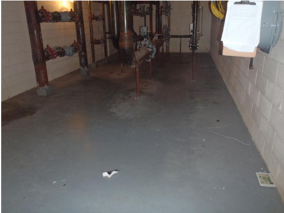
Photograph No. 7: View of cellar floor in the gas meter room of River Place II.
