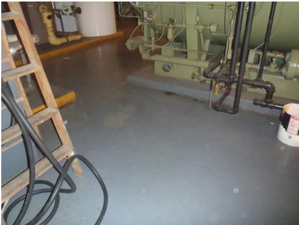
Photograph No. 16: View of concrete floor in mechanical room of River Place I.
