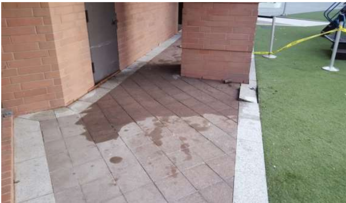
Photograph 1: View of No.2 fuel oil staining on paving stone walkway outside of pump room.
