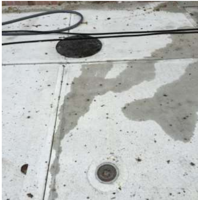
Photo 19: Fill port on 41 st Street sidewalk.
