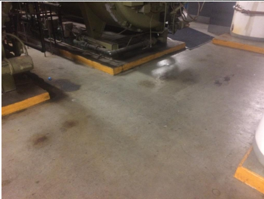
Photo 11: Surface cover in Site boiler room.
