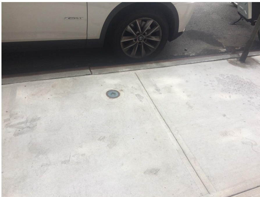
Photo 20: Fill port on 41 st Street sidewalk.
