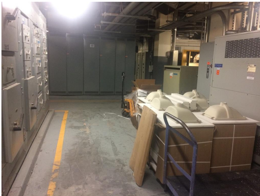
Photo 8: Surface cover in Site electrical room.
