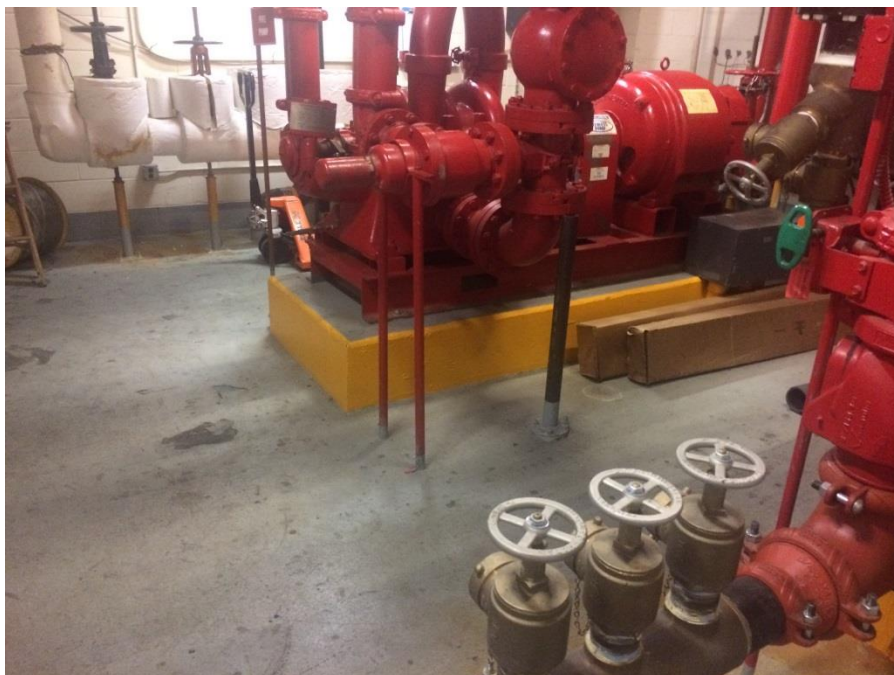
Photo 10: Surface cover in Site fire pump room.
