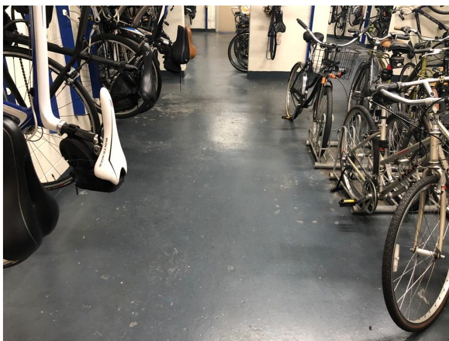
Photo 6: Ground cover in the bicycle storage room of the Site.
