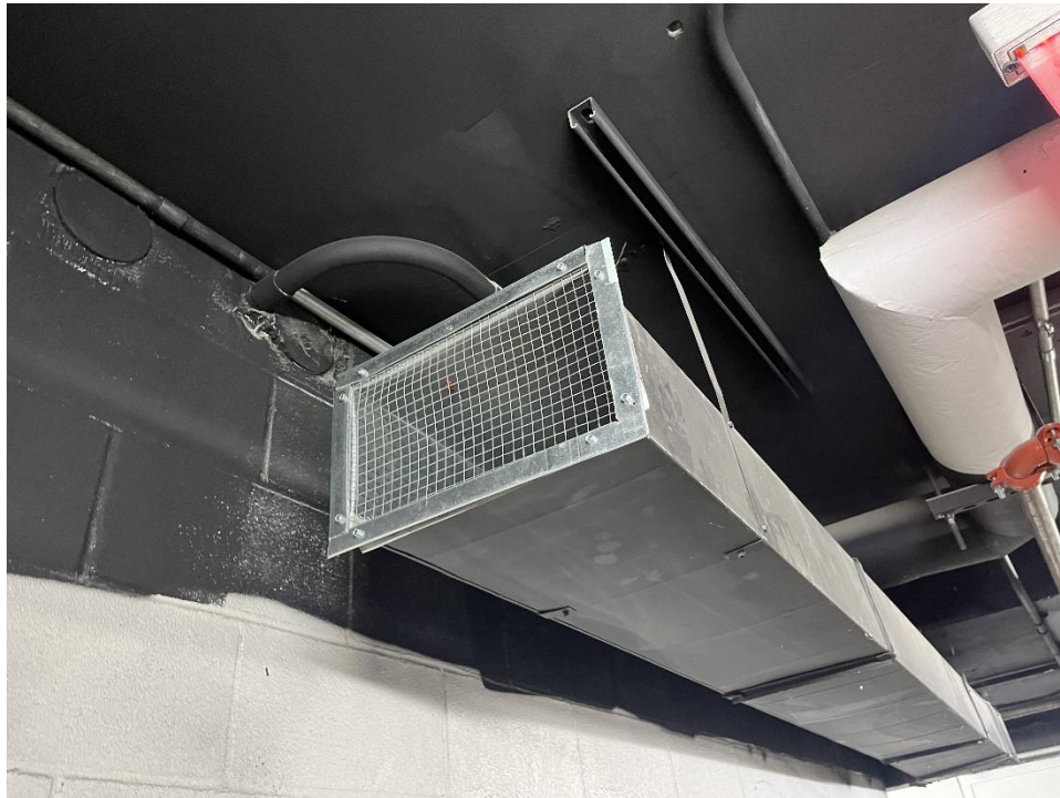
Photograph 11: Ventilation system in the parking garage (facing west).
