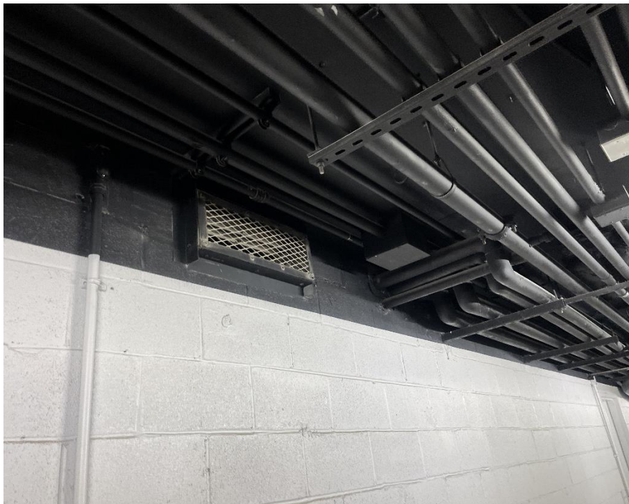
Photograph 12: Ventilation system in the parking garage (facing east).
