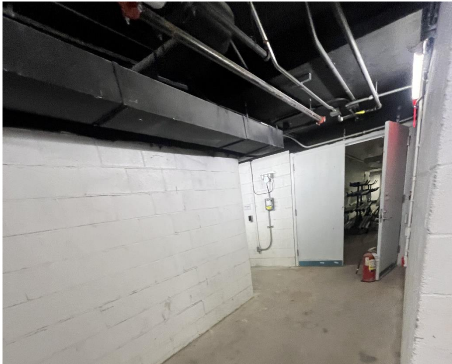
Photograph 14: Ventilation ductwork (facing south).
