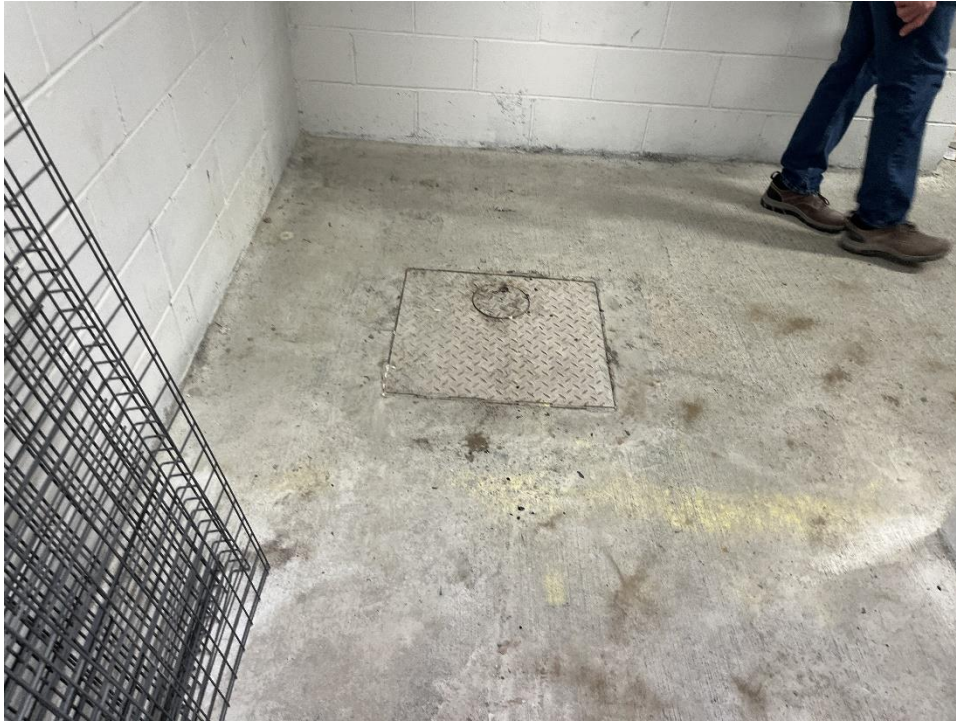
Photograph 7: Typical recovery well vault (RW-K, facing north).
