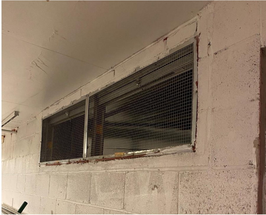
Photograph 13: Ventilation system in the parking garage (facing west).
