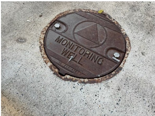
Photo 3: Typical monitoring well in active area of the Site.
