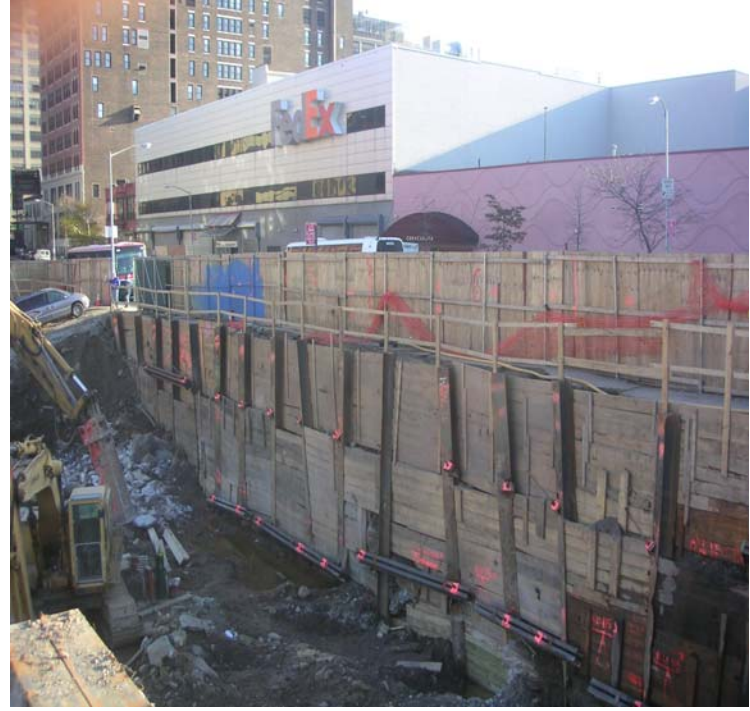
Photo 22: Lagging and sheeting along the southern wall (34 th Street), second row of tie-backs completed.
