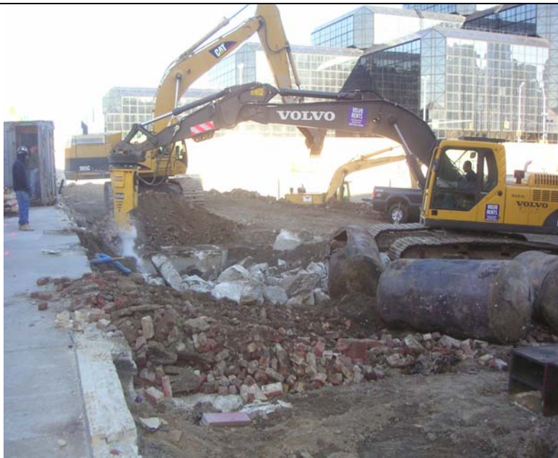
Photo 3: Breaking up for concrete vault surrounding USTs near southern gate (34 th Street).
