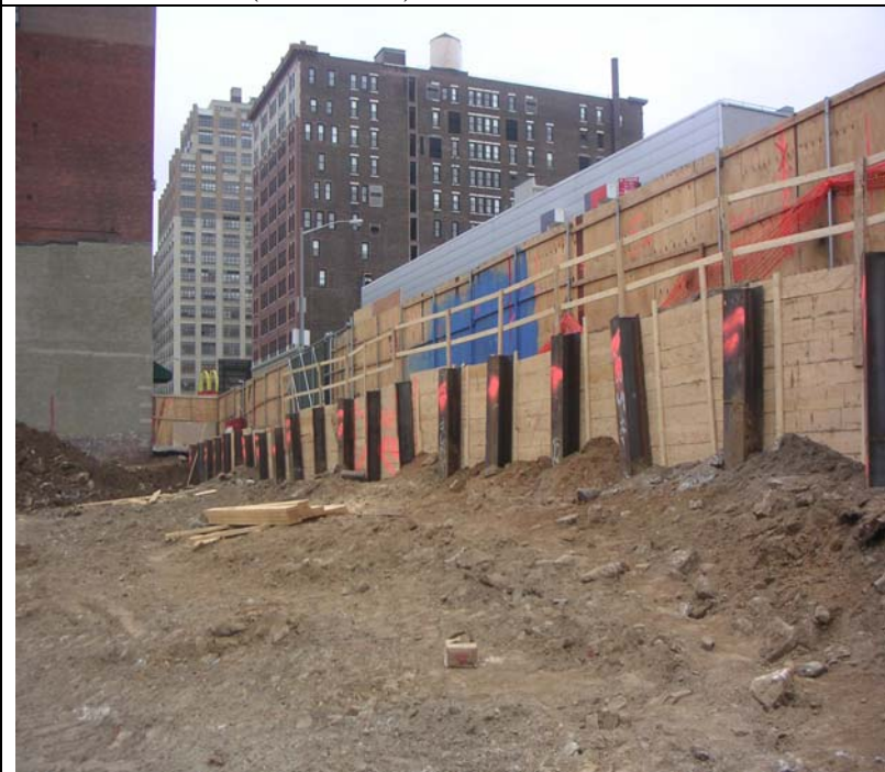
Photo 11: First stage of soldier beams and lagging along southern border (34 th Street).
