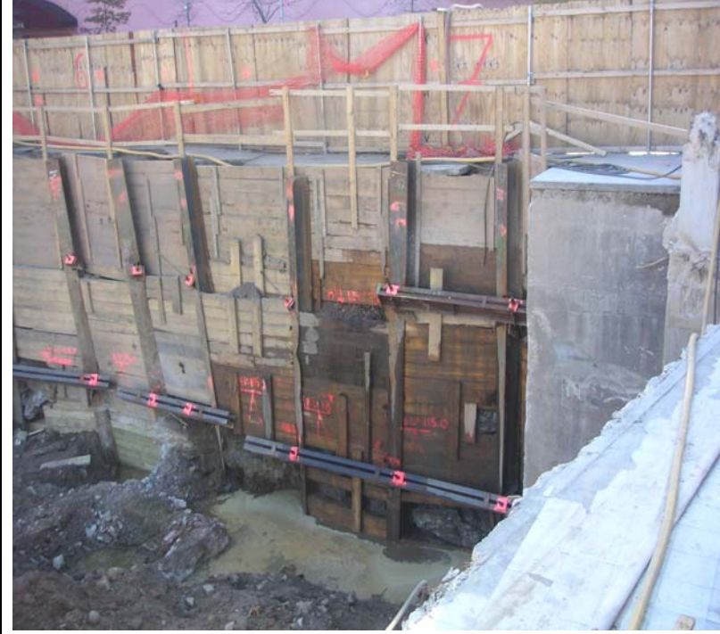
Photo 21: Incoming water in southwest corner from leaking fire hydrant on 34 th Street
