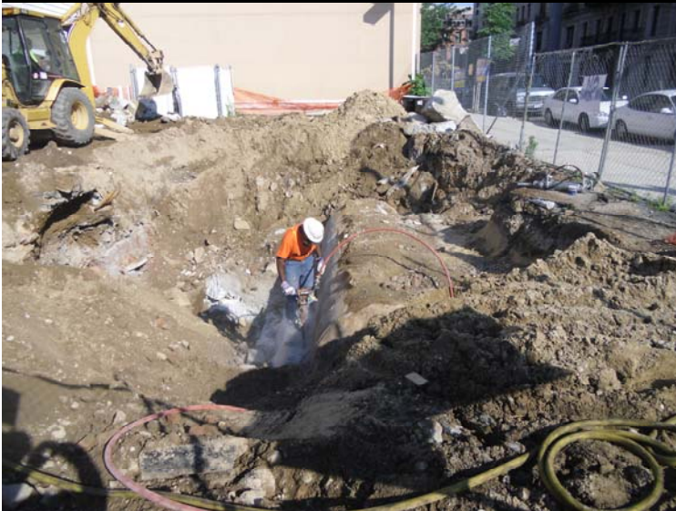
Photo 2 – 4K tank encased in concrete
