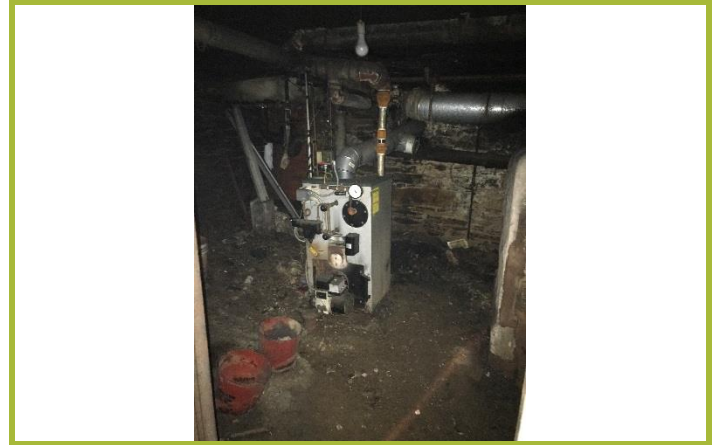
Photo #14: Additional boiler room located in the eastern section of the basement.
