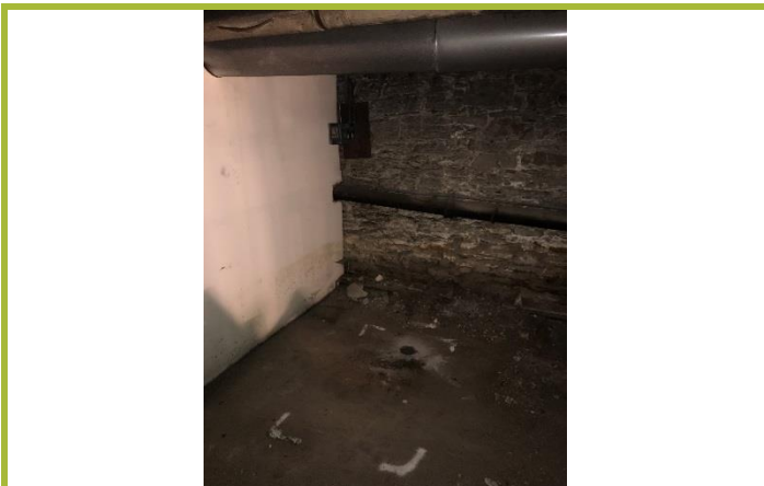
Photo #11: VTX-07 located in the basement.
