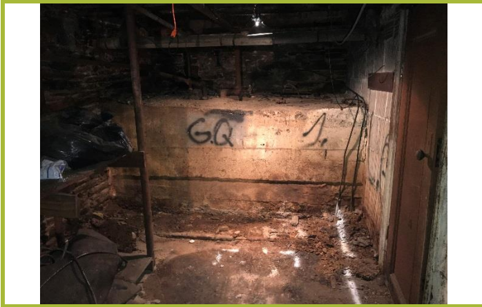
Photo #13: VTX-06, AST Soil Pile Waste Class, and vaulted AST(s) located in the rear section of the basement.
