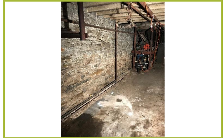
Photo #8: VTX-05 located in the basement.
