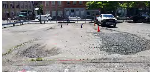
Photo 2. Surface depression in western portion of site
