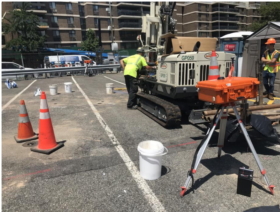
Photo 1: AARCO advancing soil boring SB4E2 in the northern part of the site (facing north)
