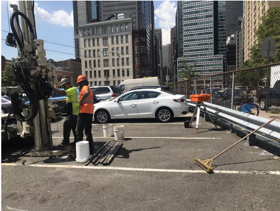
Photo 1: AARCO advancing soil boring SB24 in the northern part of the site (facing southwest)
