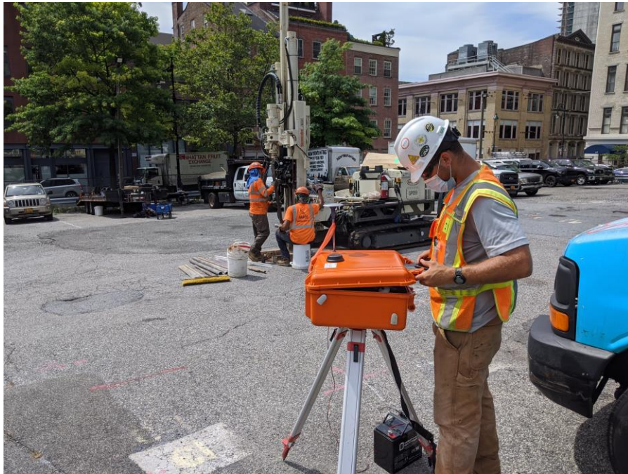
Photo 3: View of Langan checking air monitoring station WZ-1 while AARCO advances soil boring SB16 (facing south)
