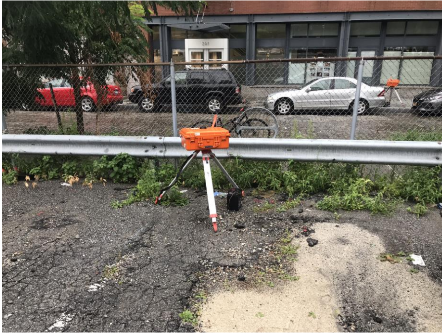
Photo 3: Work zone station WZ-1 and perimeter station PM-4 while AARCO advances boring SB-23 (facing south)
