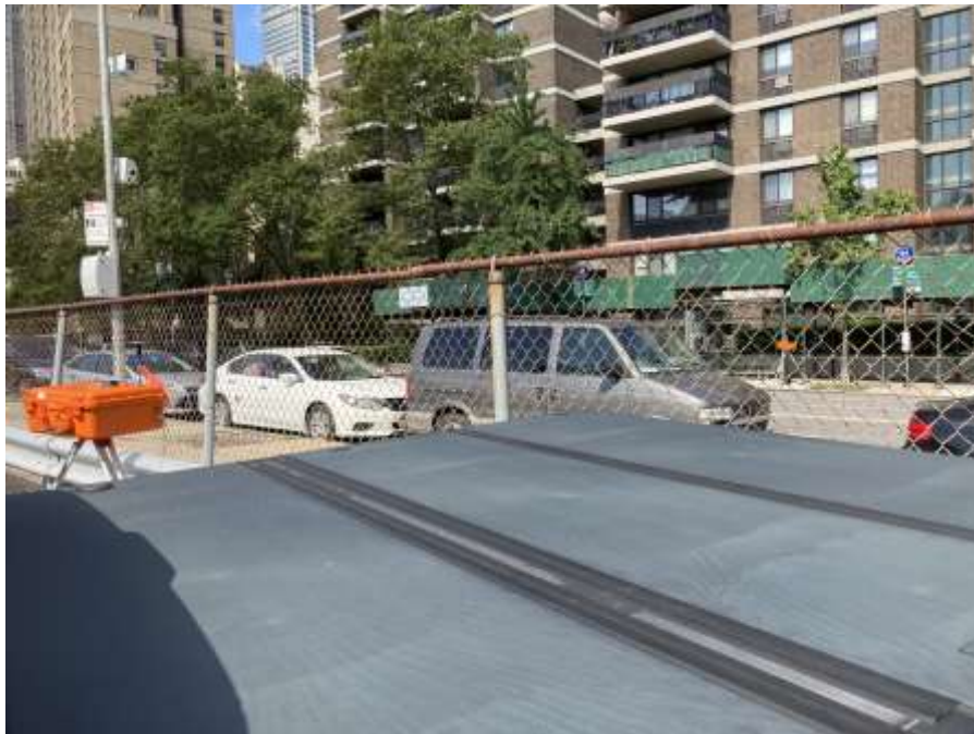
Photo 2: Perimeter CAMP station PM-4 and off-site CAMP station WZ-1 along Pearl Street during the drilling of boring SB29 (facing west).
