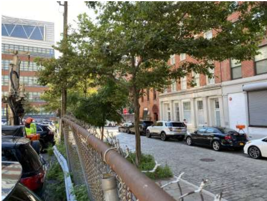
Photo 2: Perimeter CAMP station PM-6 and off-site CAMP station WZ-1 along Water Street during the drilling of boring SB28 (facing east).
