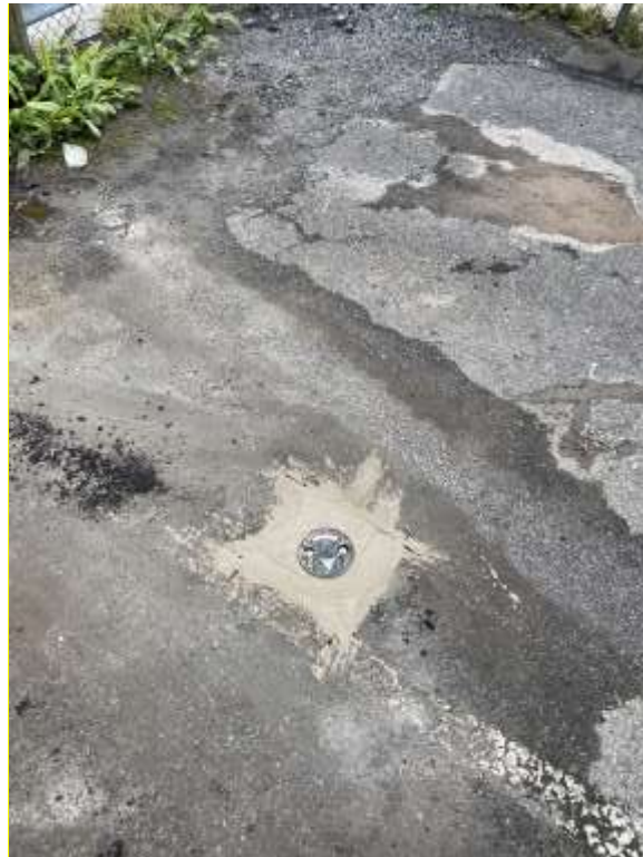
Photo 4: View of monitoring well MW11.
