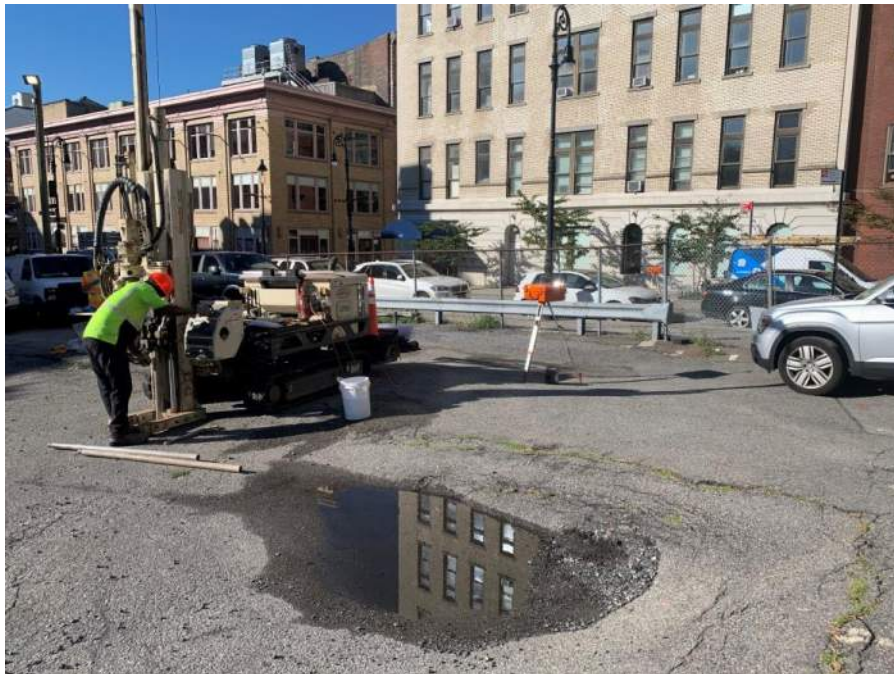
Photo 2: Perimeter CAMP station WZ-1 and off-site CAMP station PM-2 along Beekman Street during the drilling of boring SB37 (facing southwest)
