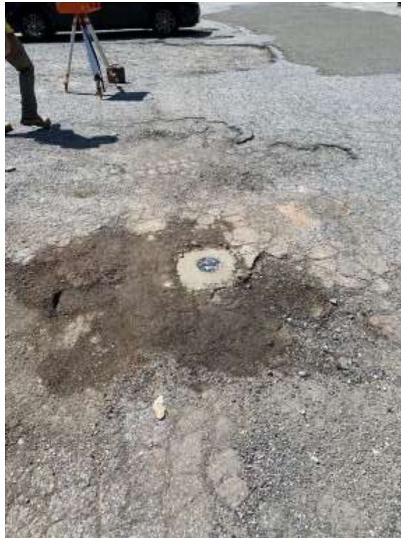
Photo 4: View of installed MW26 (facing southwest)
