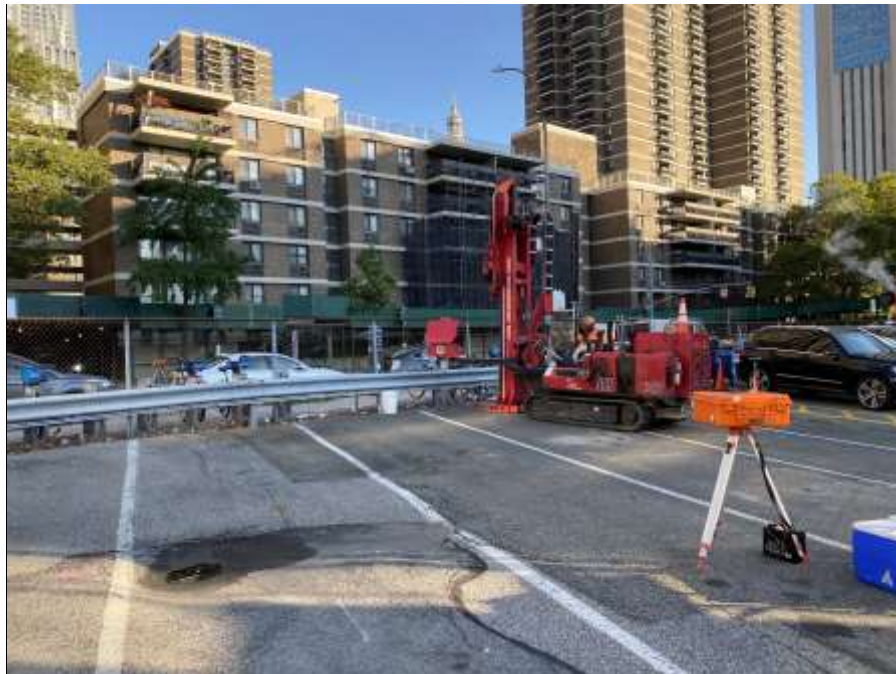
Photo 2: Perimeter CAMP station WZ-1 and off-site CAMP station PM-4 along Pearl Street during the drilling of boring SB4N3 (facing north)
