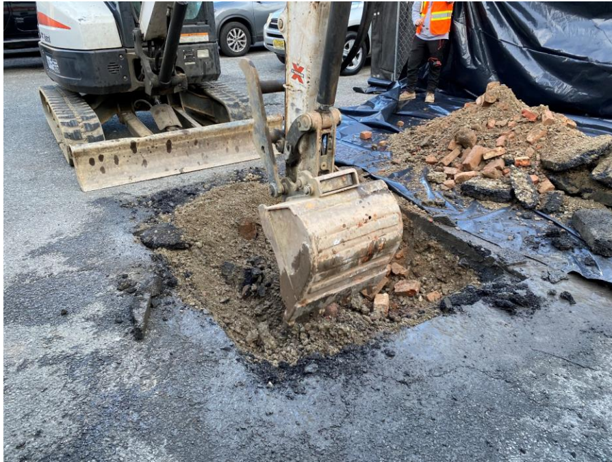
Photo 3: View of AARCO excavating test pit TP03 and stockpiling excavated soil/fill on polyethylene sheeting (facing southeast).
