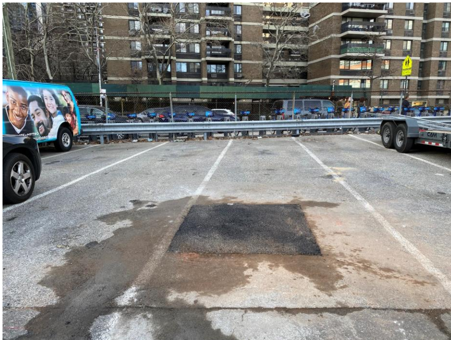
Photo 4: View of test pit TP05, restored to the surrounding grade using cold patch asphalt (facing north).
