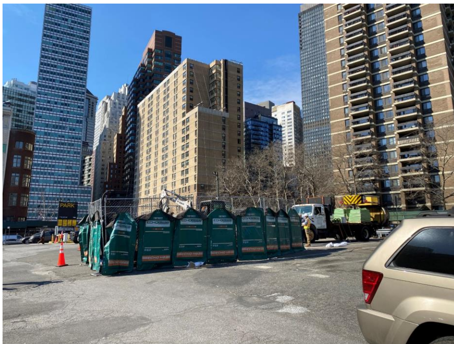
Photo 2: View of typical work zone fencing with chain-link fence and Echo Barrier H9™ acoustic curtains (facing northwest).
