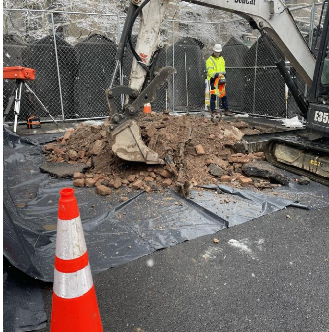
Photo 3: View of Jerome® J505 screening during backfilling of Test Pit TP04 (facing north)
