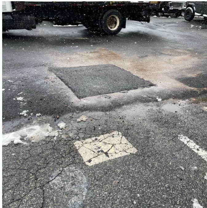
Photo 4: View of test pit TP04, restored to the surrounding grade using cold patch asphalt (facing north).
