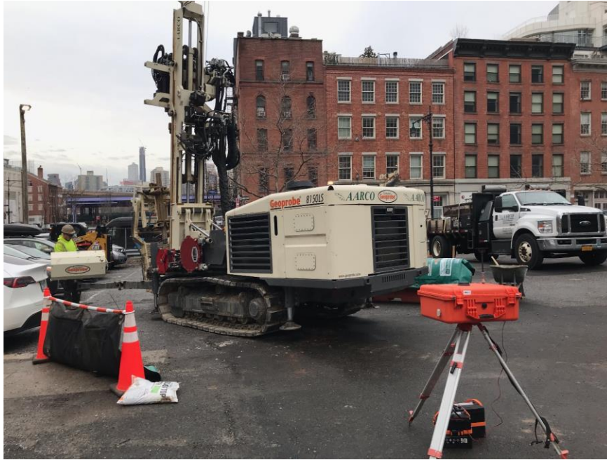
Photo 1: View of AARCO advancing a soil boring in the southeast part of the site (facing south).
