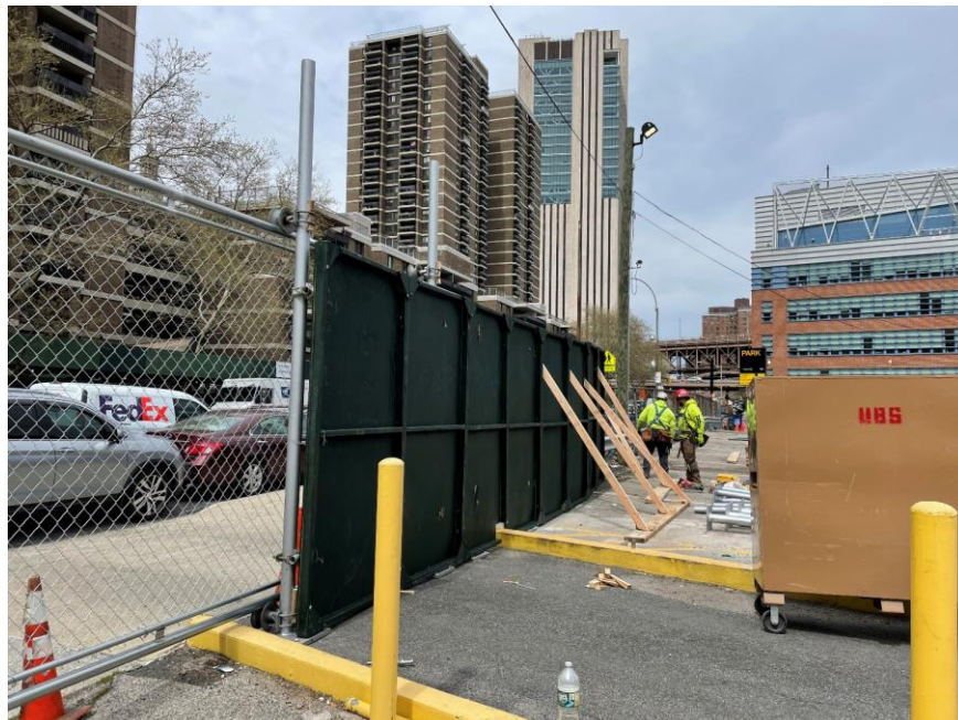
Photo 2: UBS installing construction fence at the northern perimeter of the site (facing northeast)
