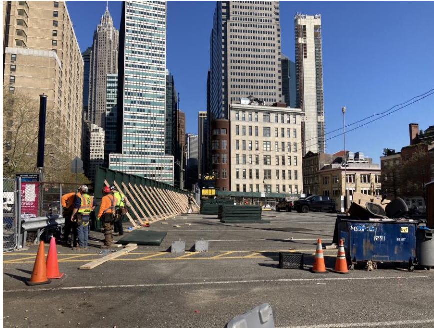
Photo 1: View of perimeter construction fencing installed along the northern boundary of the site (facing west).
