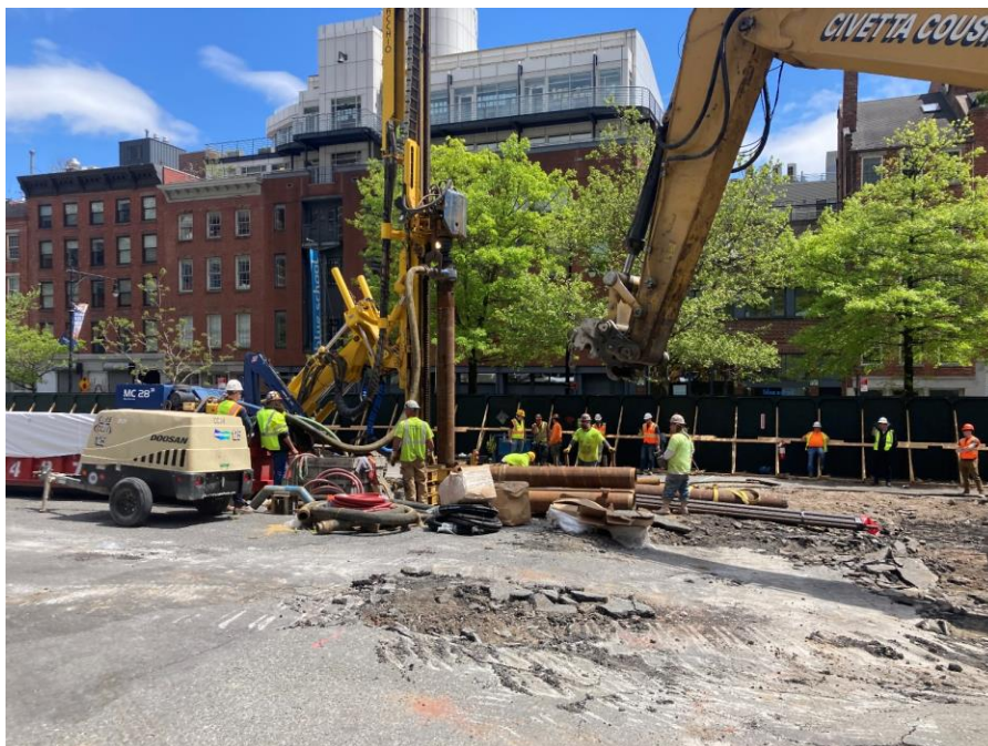
Photo 2: CCJV advancing a pile in the southwestern portion of the site (facing south)
