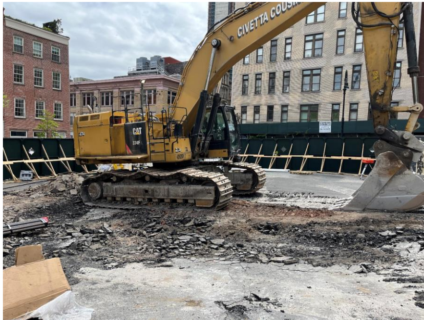
Photo 1: CCJV removing the asphalt cover in the southwestern portion of the site (facing southwest)
