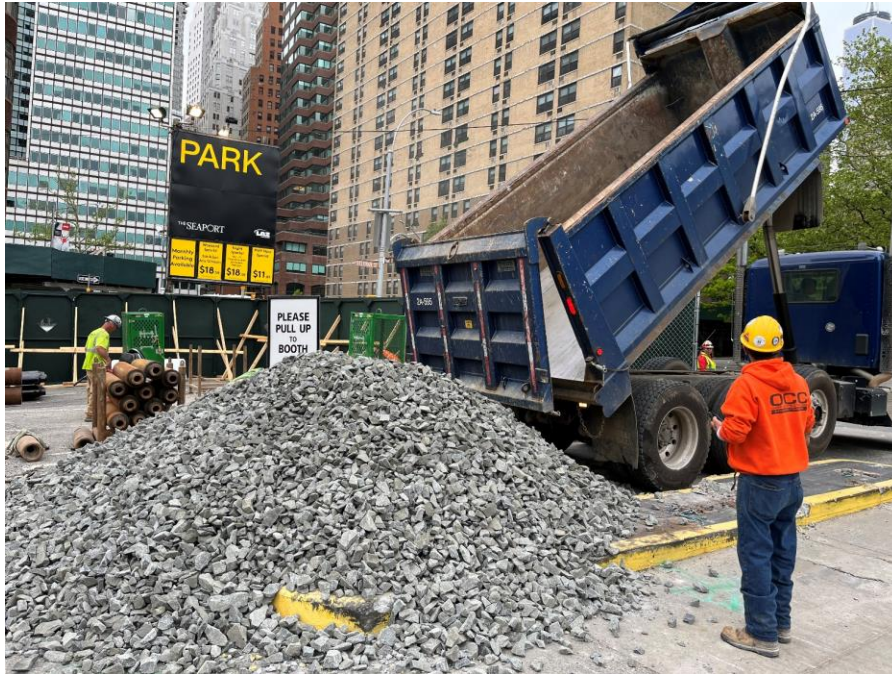
Photo 1: CCJV importing one truckload of 2.5-inch virgin stone for installation of a tracking pad in the northwestern portion of the site (facing northwest)
