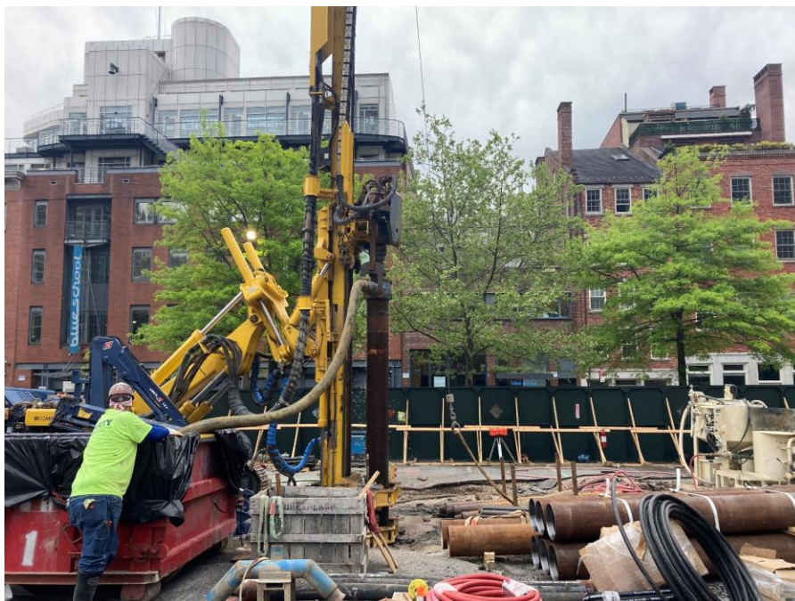
Photo 2: View of CCJV advancing a pile in the southwestern portion of the site (facing south)
