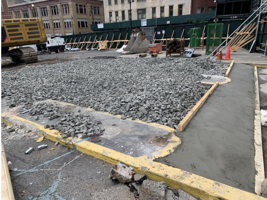
Photo 1: View of concrete placed along the northern edge of the tracking pad (facing southwest).
