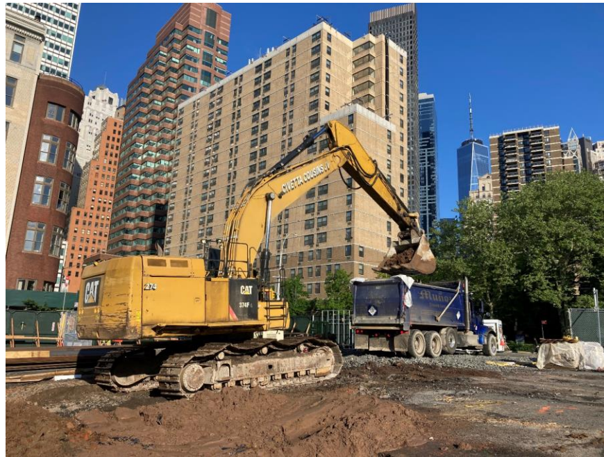
Photo 1: View of CCJV live-loading a permitted, tri-axle truck with hazardous lead-impacted soil/fill for off-site disposal (facing northwest)
