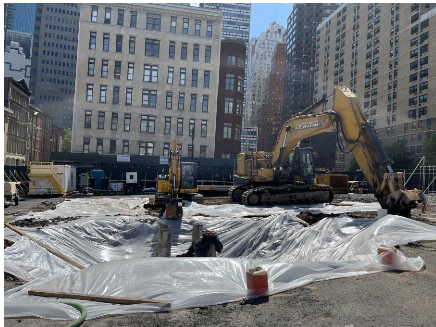
Photo 2: View of the covered excavation area at the end of the work day (facing south)
