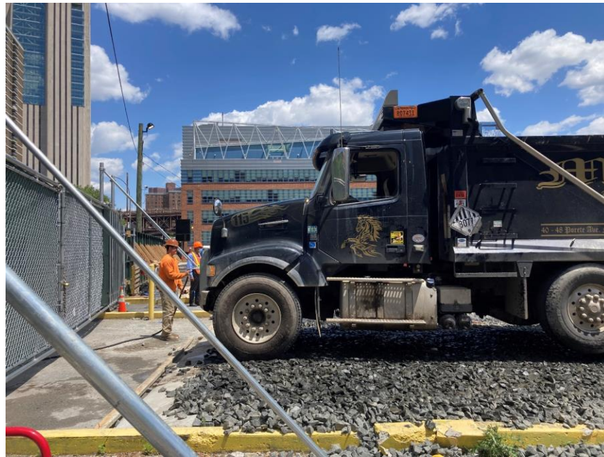
Photo 3: View of CCJV washing a truck prior to exiting the site (facing east).
