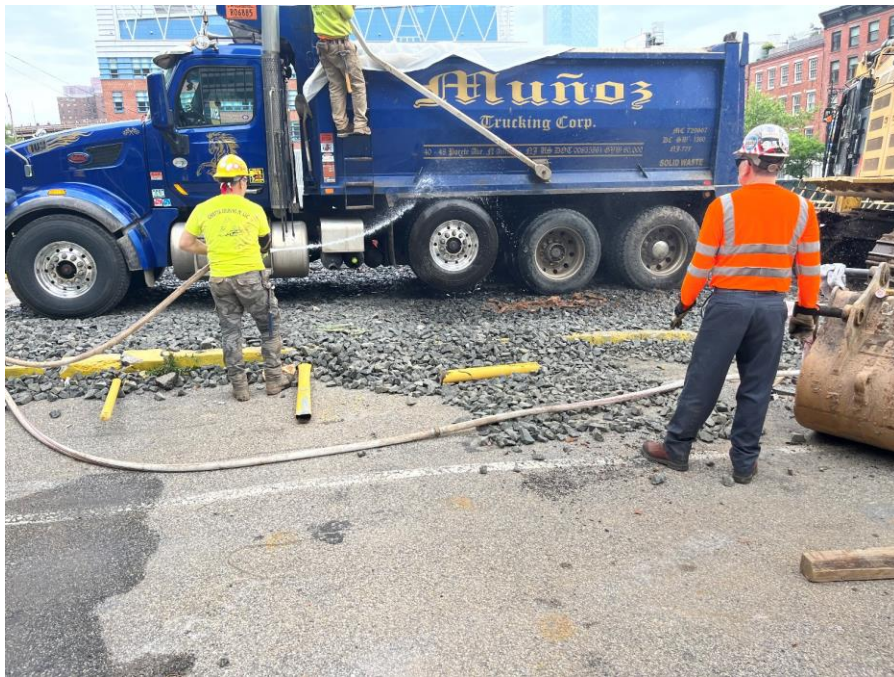
Photo 1: View of CCJV washing a truck prior to exiting the site (facing east)
