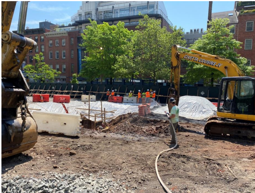
Photo 1: View of CCJV implementing dust suppression measures in the southwestern portion of the site (facing south)
