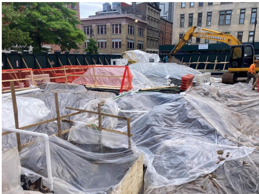
Photo 2: View of exposed soil/fill and imported virgin stone stockpiles covered at end of day (facing southwest).
