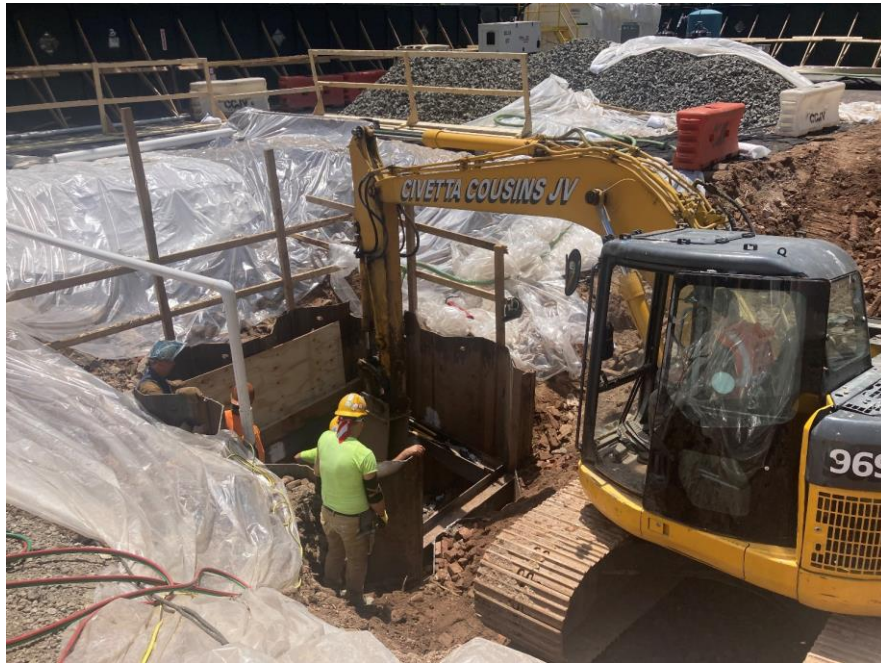
Photo 1: View CCJV excavating soil/fill between previously installed foundation piles in the southwestern portion of the site (facing southwest)
