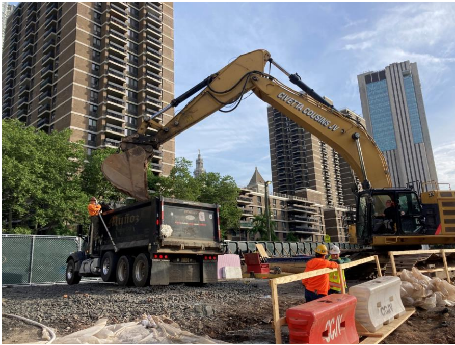
Photo 1: View CCJV loading a truck with hazardous lead-impacted soil/fill for off-site disposal (facing northeast)
