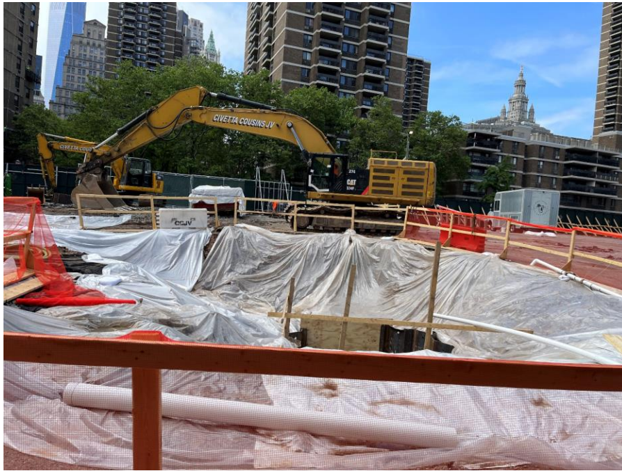
Photo 3: View of exposed soil/fill covered with polyethylene sheeting at the end of the day (facing north)
