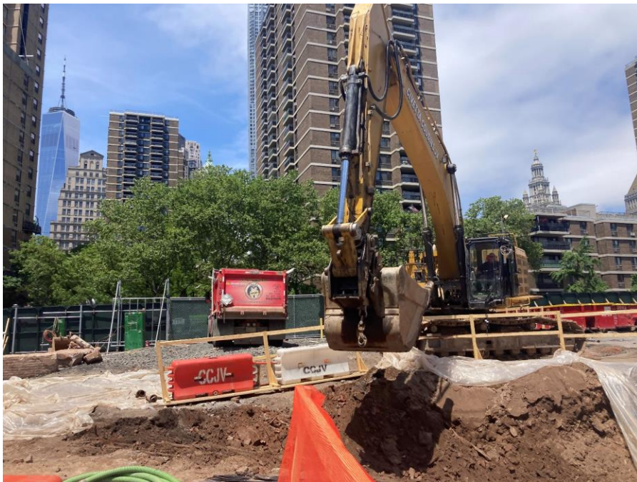
Photo 2: View of CCJV excavating hazardous lead-impacted soil/fill along the northern berm of the work area in the southwestern portion of the site (facing north)
