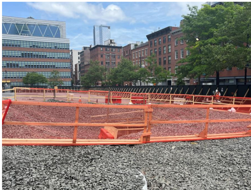
Photo 2: View of the work area in the southwestern part of the site, covered with geotextile fabric and imported 2.5-inch virgin stone (facing southeast).
