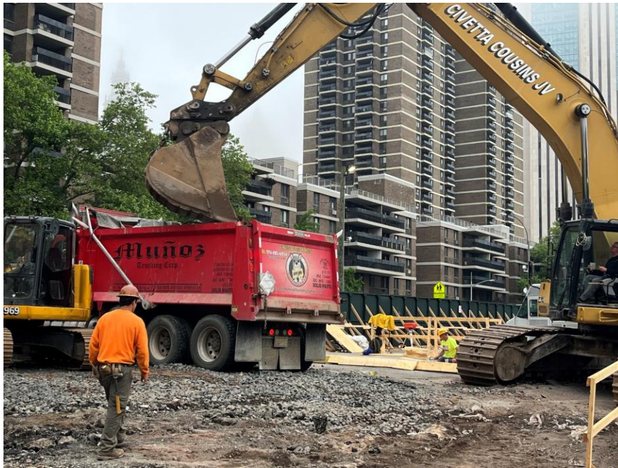
Photo 1: View of CCJV live-loading a truck with hazardous lead-impacted soil/fill for off-site disposal at the CENJ facility, located in Kearny, NJ (facing northeast).
