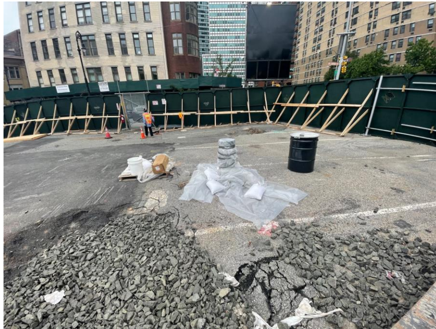
Photo 3: View of the installed test pile covered with polyethylene sheeting in the northwestern part of the site (facing west)
