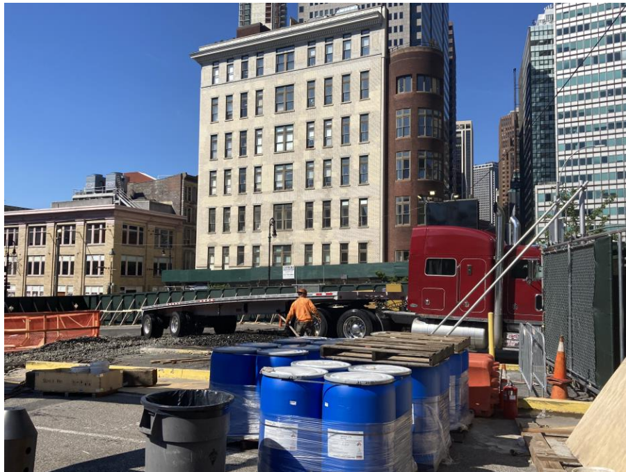
Photo 1: View of staged 55-gallon drums containing Atmos® AC-645 dust/odor suppressing foam (facing west)
