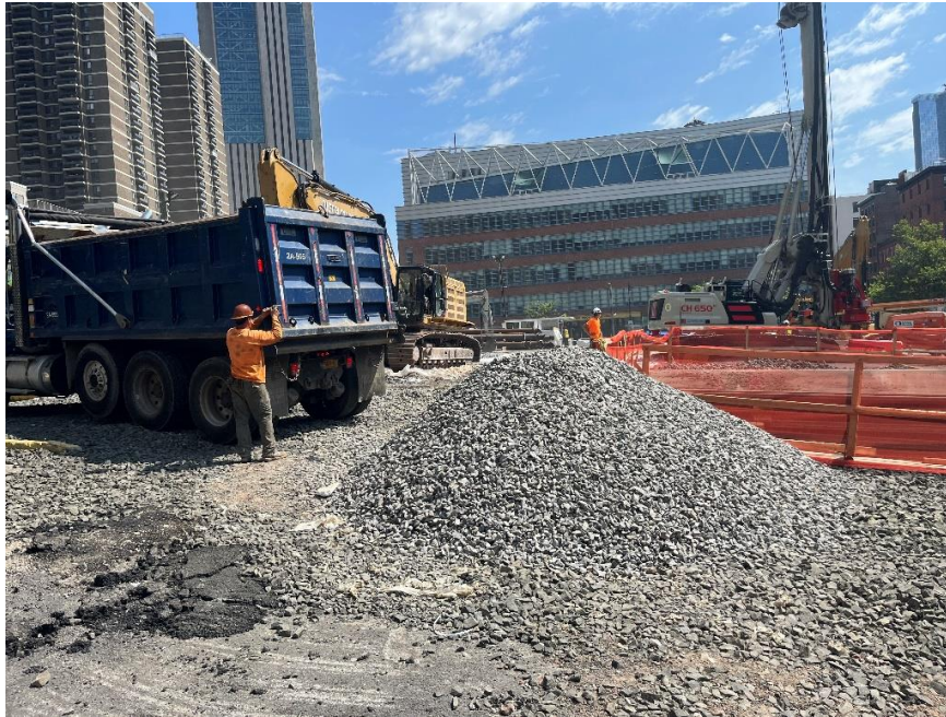
Photo 1: CCJV importing 1.5-inch clean bluestone to extend the truck tracking pad in the northwestern part of the site (facing east)
