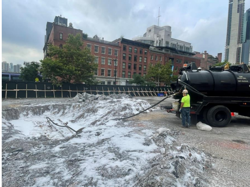
Photo 1: Brookside removing petroleum product/water mixture from a previously identified UST in the eastern part of the site (facing southwest)
