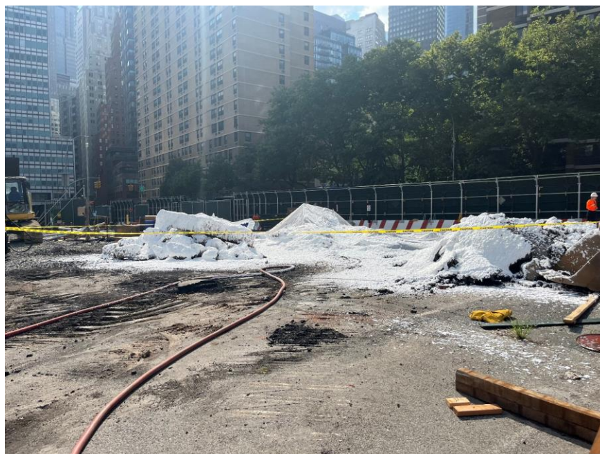
Photo 2: View of the excavation area in the north-central part of the site covered with polyethylene sheeting and/or Atmos® AC-645 dust/vapor suppressing foam (facing northwest)
