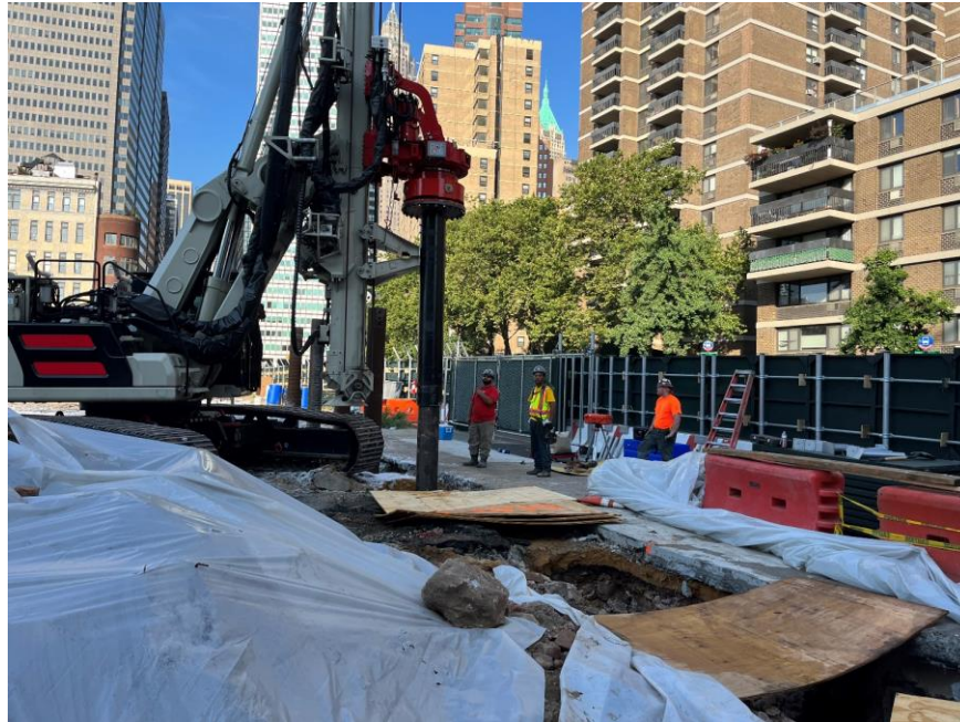
Photo 1: CCJV installing SOE soldier piles along the northern boundary of the site (facing northwest)
