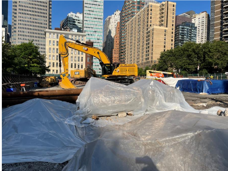
Photo 3: View of the four USTs placed on and covered with polyethylene sheeting (facing northwest)
