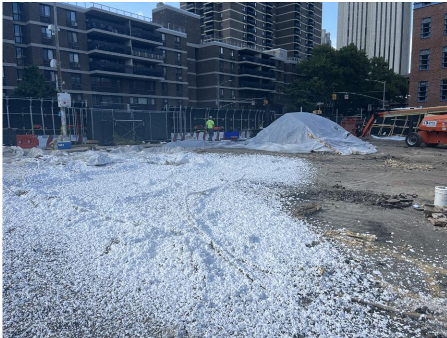
Photo 1: Exposed soil/fill and stockpiles covered with Atmos-AC-645 dust/vapor suppressing foam and/or polyethylene sheeting (facing northwest)
