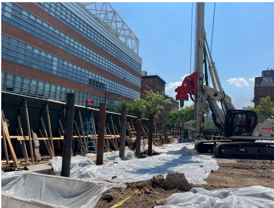
Photo 2: CCJV installing SOE soldier piles along the eastern boundary of the site (facing southeast)
