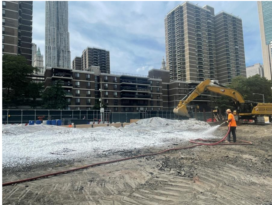
Photo 3: CCJV applying Atmos ® AC-645 dust/vapor suppressing foam to create a temporary overnight cover at the end of the work day (facing northeast)
