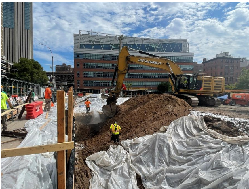
Photo 2: CCJV excavating soil/fill in the north-central part of the site and actively applying Mercon-X® (facing northeast)
