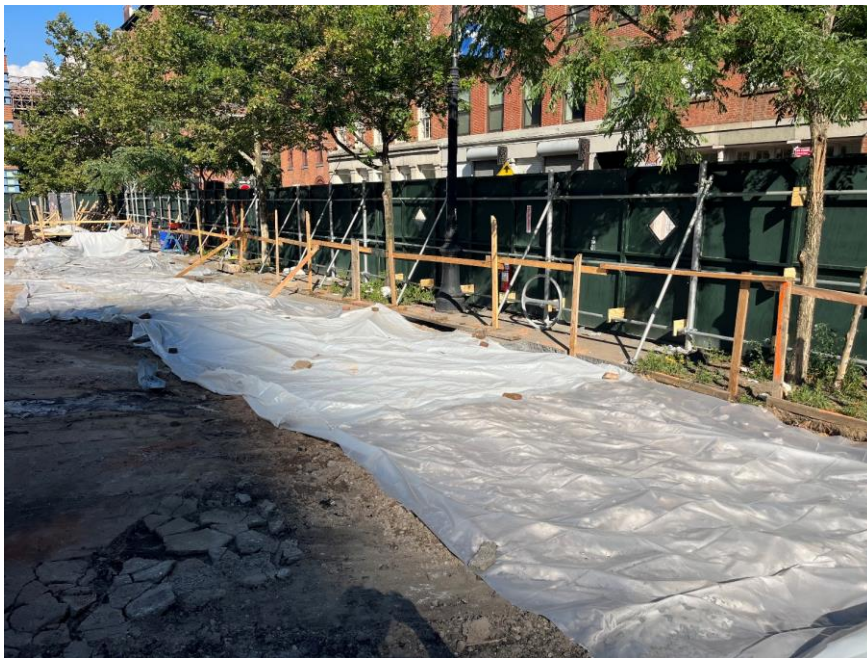
Photo 2: Exposed soil/fill covered with polyethylene sheeting along the southern site boundary (facing southeast)
