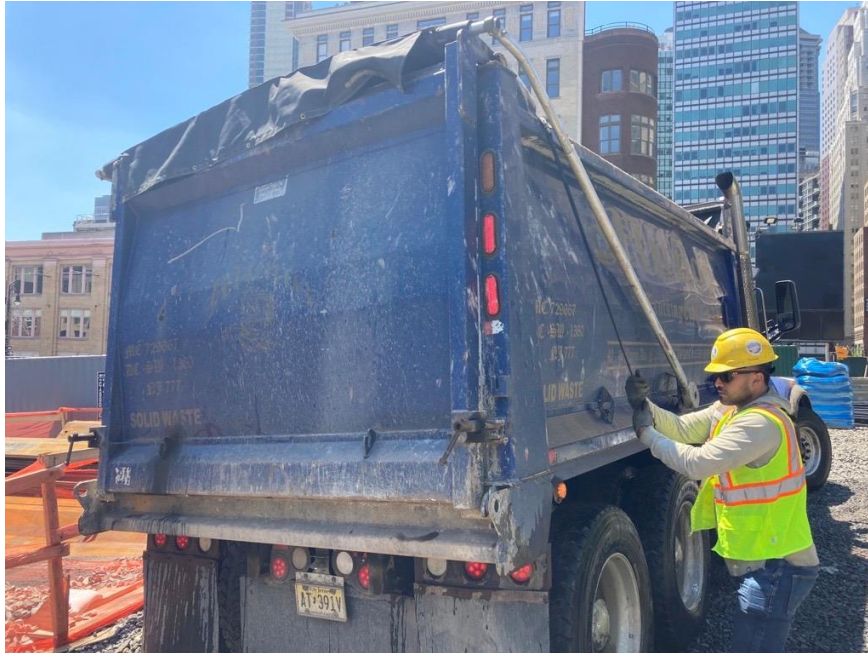
Photo 3: CCJV securing a tight-fitting cover to a loaded dump truck prior to exiting the site (facing west)
